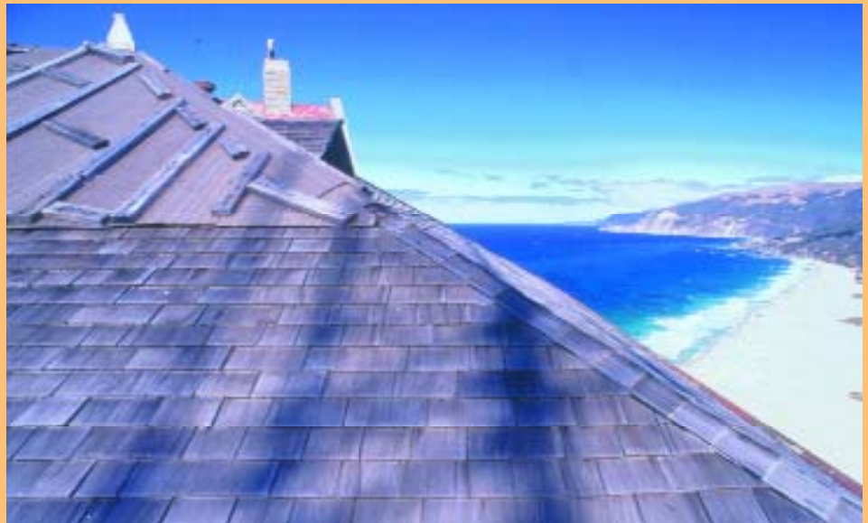
Before and After: State Park deferred maintenance funds were used to replace a roof at Point Sur SHP.
