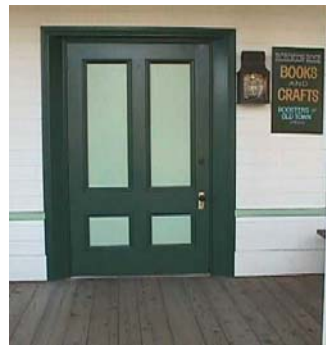
At the Robinson Building, a single door, rather than commercial double doors with glass, was installed.
