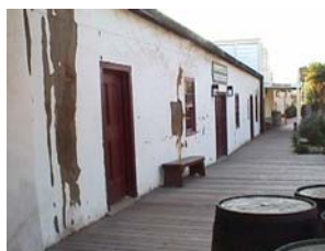
Poor restoration work in the 1960s has created continual maintenance problems for the adobe.
