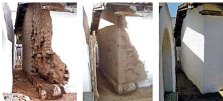
Stabilization of the adobe walls of El Cuartel was completed in 2002 with funding from the department's Cultural Stewardship Fund.
