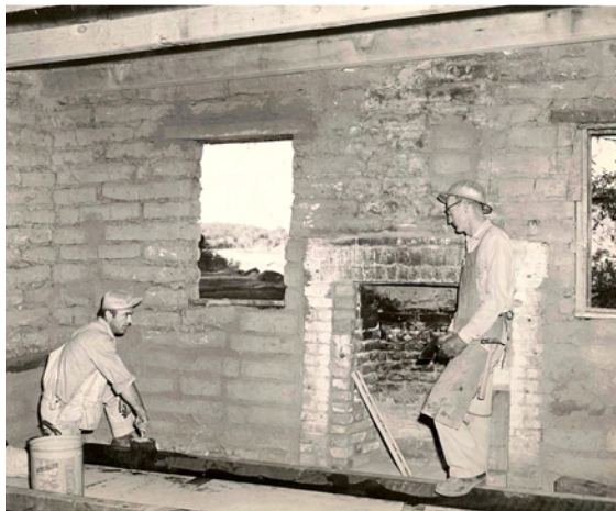
Interior view of the rehabilitation work on the Adobe. California State Parks Collections.
