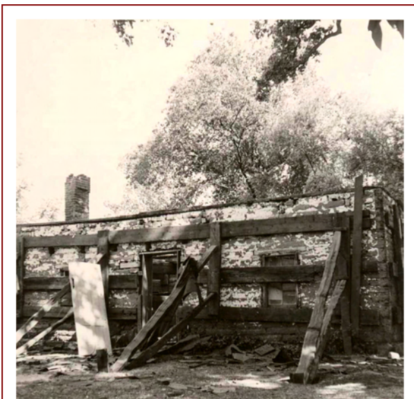
The Adobe after the roof was removed in July 1958. California State Parks Collections.
