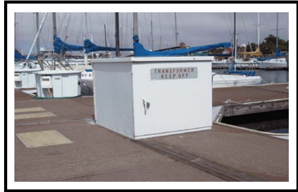
Dead Load on a Dock: Electrical Transformer Cabinet
