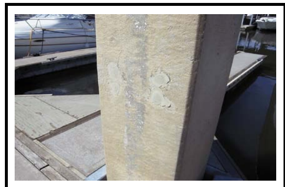
Rough Face on Square Concrete Pile
