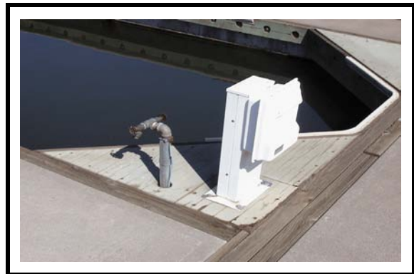
Power Center and Separate Water Supply
