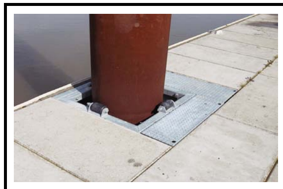
UHMW Rollers on Round Steel Guide Pile
