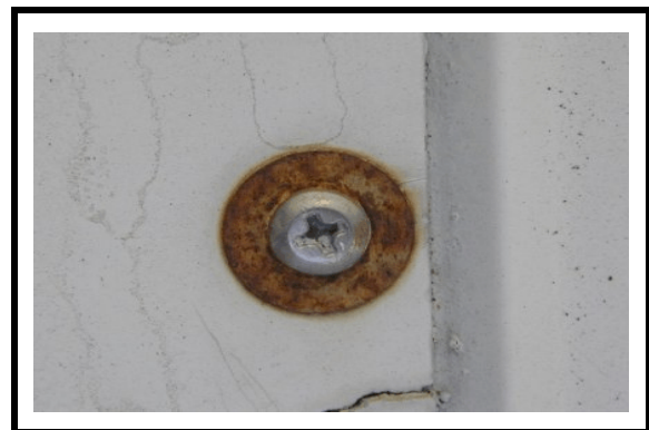
SS Screw and Corroded Cadmium-Coated Steel Washer
