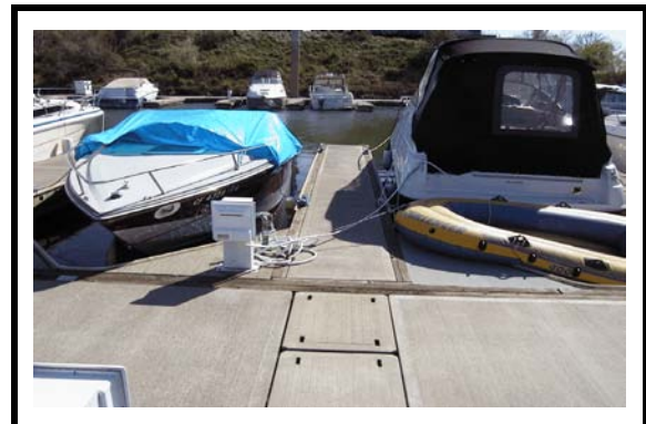
Non-Permanent Utility Lines Across Fingerfloat
