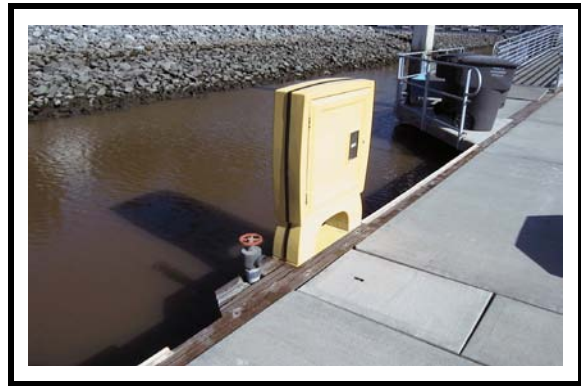
Dock-Side Fire Hose Cabinet
