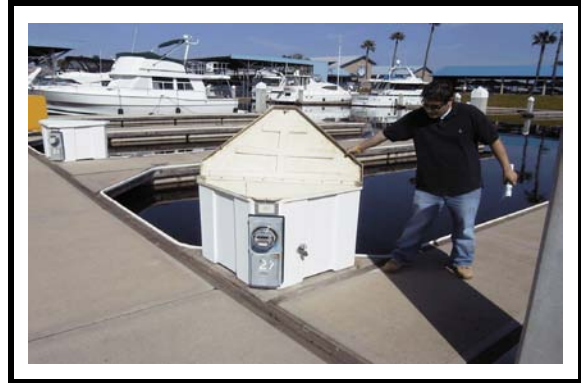
Storage Box with Power & Water Supply
