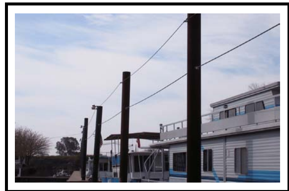
Marina Pile-Cable Restraint System
