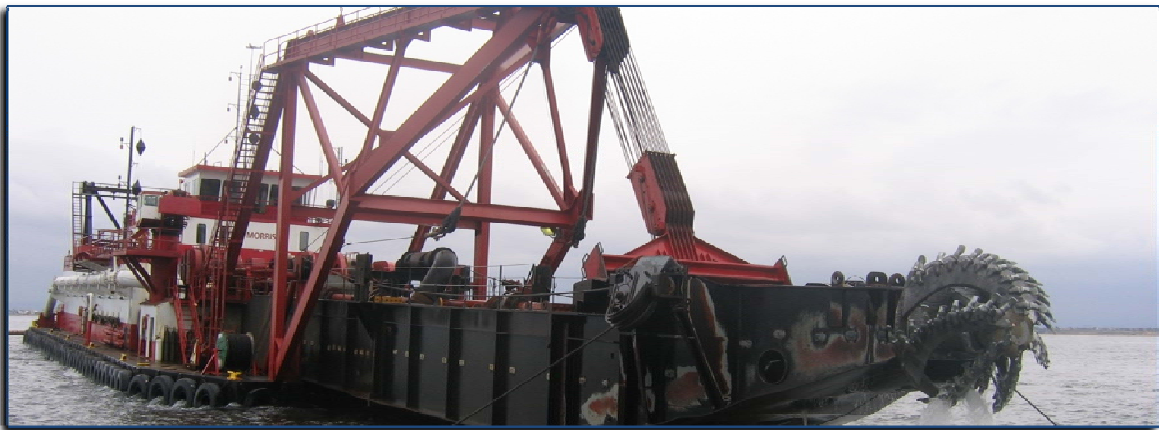
Bulldozer (top) and a dredge (above) work to restore beach sand along the Orange County coast
