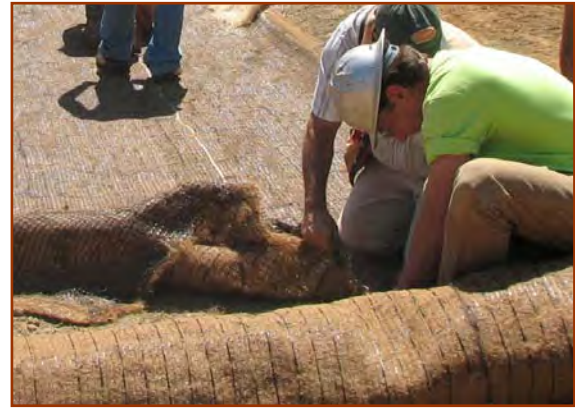
A coir composite TRM being installed and anchored into a check slot.
