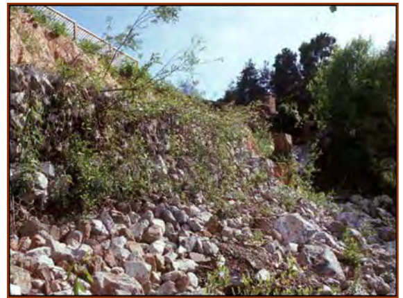
Vegetated gabions after only 4 months (Branciforte Creek in Santa Cruz County). The willow poles were inserted through the baskets during construction, then backfilled with rock. (J. McCullah photos)
