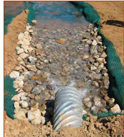
RC-1 Energy Dissipator.
