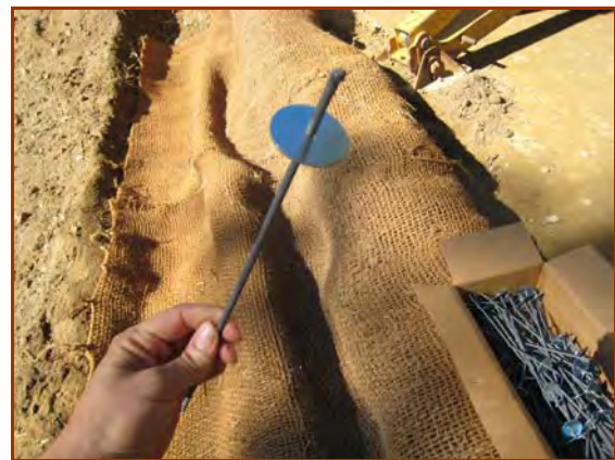
Metal stake pins with steel washers may be used for anchoring ECBs.
