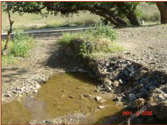
A 2001 Caltrans study (Racine and Hoover, 2001) indicated gabions last an average of 15 years until succumbing to the effects of corrosion and abrasion.
