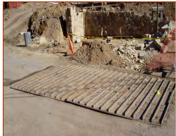
Portable rumble strips are made from plate steel and angle iron. Rumble strips are suited for construction entrances/exits where rock alone is insufficient.
