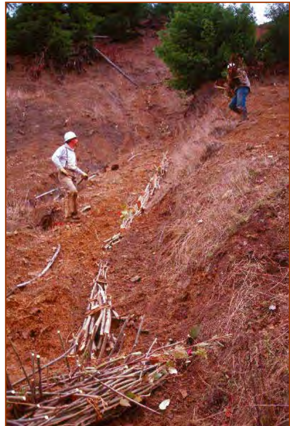
The gullies were packed with Live Pole Drains (Live Fascines) to allow subsurface drainage.
