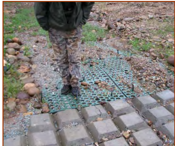
Scour Stop ® can be vegetated. Here it is used for outlet transition and channel protection. (J. McCullah photos, 2006)
