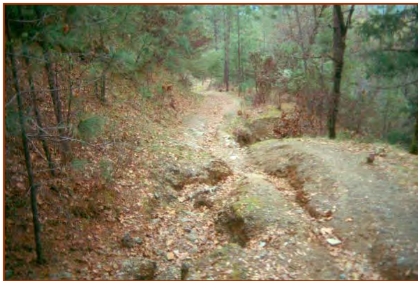
The gully causing runoff on this road/trail can be dispersed by outslipping the trail.
