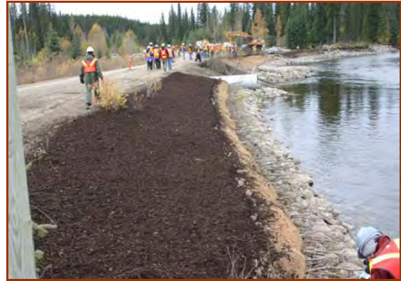
Compost blanket at vanes 2 and 3. Note that willow cuttings were also incorporated into this streambank protection design. (2005)
