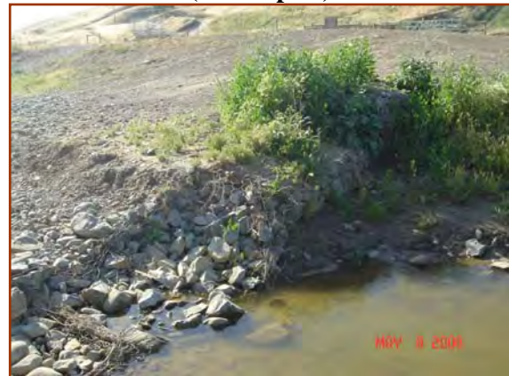
Gabion wire is abraded by stream sediment and corroded by water until the structures fail. (J. McCullah photos)
