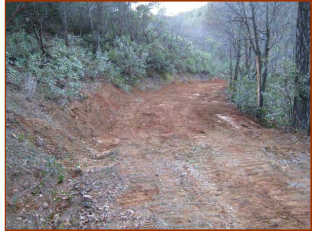
On this same road, just before the transition from inslope to outslope, a rolling dip is constructed to take runoff from the inslope section off the road.
