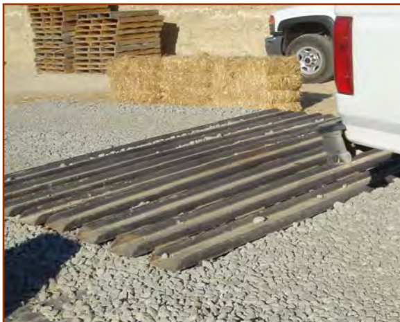
Rumble strips are steel ribs that help knock mud off and prevent tracking of mud onto highways.
