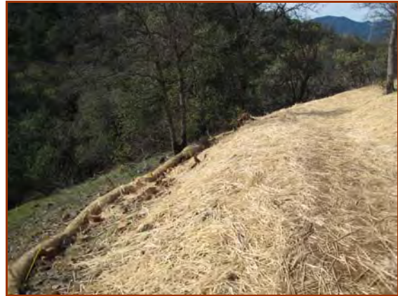
The “stake and rope method” of anchoring fiber rolls was used for sediment control along this outsloped recreational trail.
