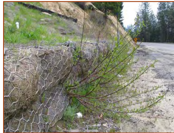
Vegetated (willow pole) gabions at the toe of a highway cutslope in Trinity Hwy 299W. The deeply planted willow pole plantings are at 3000' elevation and have survived four summer seasons (100° F plus).
