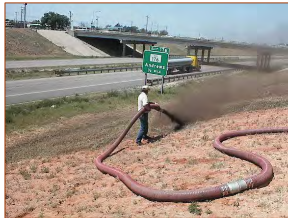
A 2 inch thick compost blanket, applied pneumatically for surface stabilization. (Photo Courtesy of Texas DOT.)
