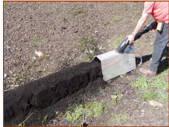
Compost berms are relatively new Best Management Practice (BMP) sediment control technology.
