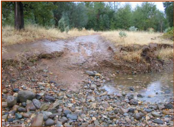
Roads entering channels should be adequately stabilized. The photo above shows no protection.
