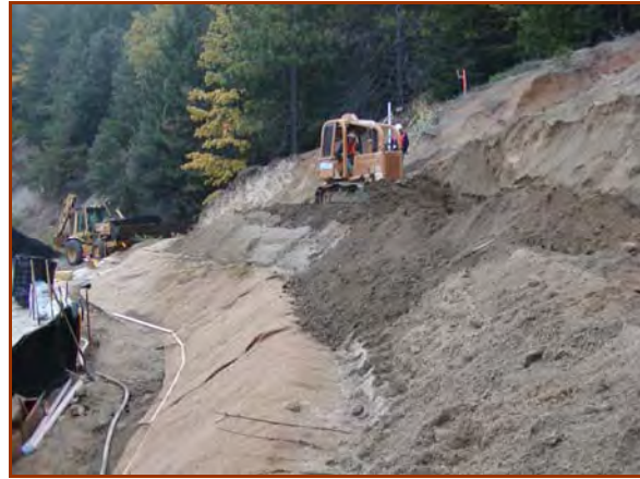
The adverse soil on this decomposed granite slope was stabilized by using a 25% compost mix.
