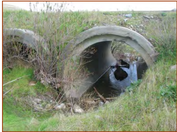
One advantage of concrete culverts is an estimated life of 75 years.
