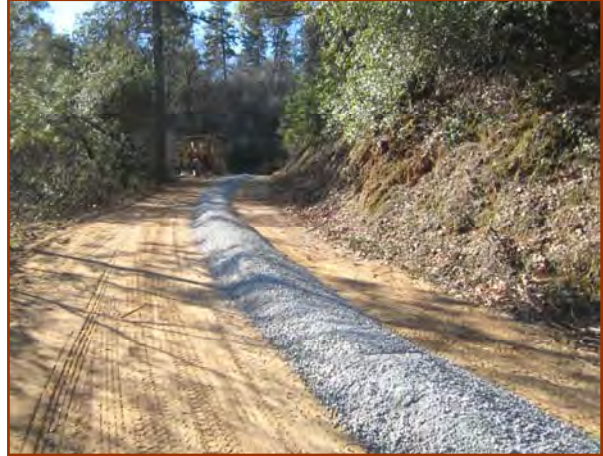
20T of base rock dumped in a downhill direction with a “bellydump” is ready for spreading.
