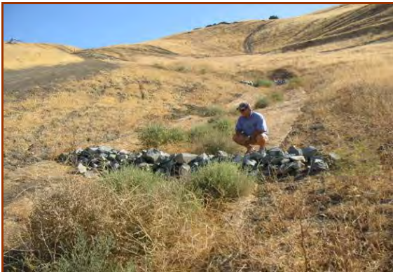
This rock check dam needs a lower weir crest to avoid "end runs".
