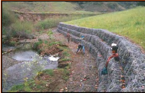
Morrow Creek, Morrow Bay, CA (March 1999). Scour apron being planted with Live Staking “after the fact”. It is very difficult to plant gabions after construction.
