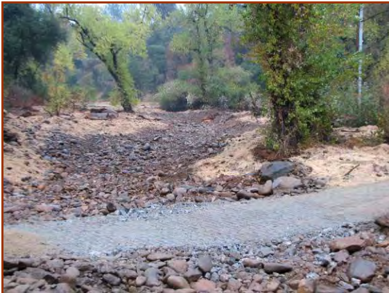
This ACB system is in-filled with ¼ inch granular aggregate to help lock blocks together.
