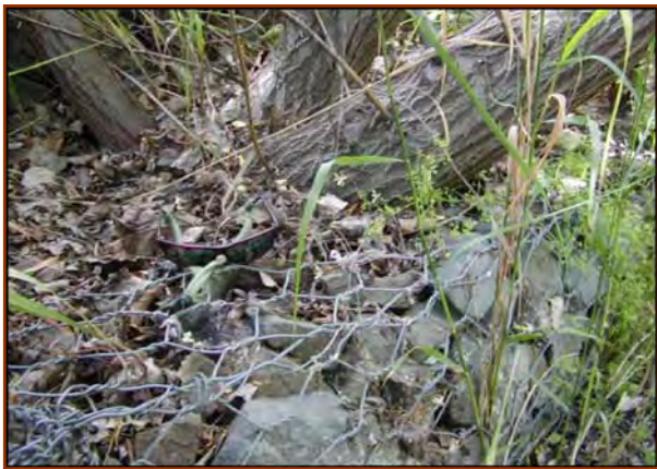
This rock-filled gabion has a 10 year-old willow tree growing through it with no deformation or “lifting”. There is ample proof that woody vegetation will only reinforce gabions, not cause structural compromise.
