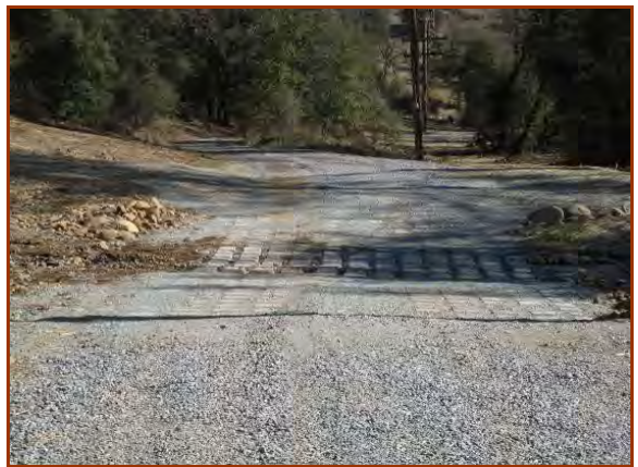
Same crossing after several winter storms and daily traffic.
