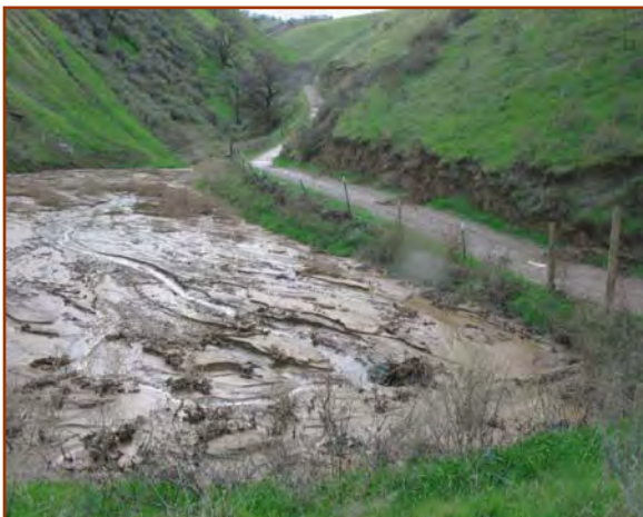
Sediment ponds need to be cleaned out prior to the rainy season, and the sediment needs to be stockpiled and properly protected.
