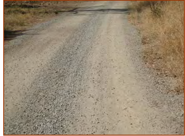
Maintenance of surfaced roads should be done annually before the rainy season.
