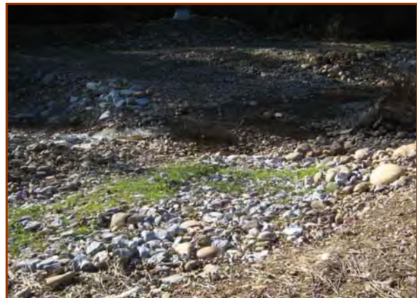
This emergency (rocked) crossing was constructed by “over-cutting” the banks 6-9 inches and laying well-compacted “gabion rock” (4-6 inch) as a structural base. The structure in the creek is a cross vane weir designed for fish passage. (J. McCullah photo, 2007)
