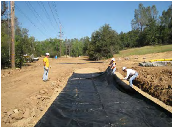
Geotextile is placed over compacted sub-base to provide stability and prevent "pumping" of fines.
