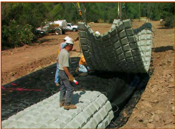
The leading edge of the cabled mat is placed in a "cut-off trench".
