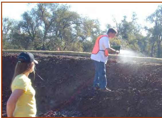
PAM is being dry-applied to a slope during trials at Shasta College (2005).
