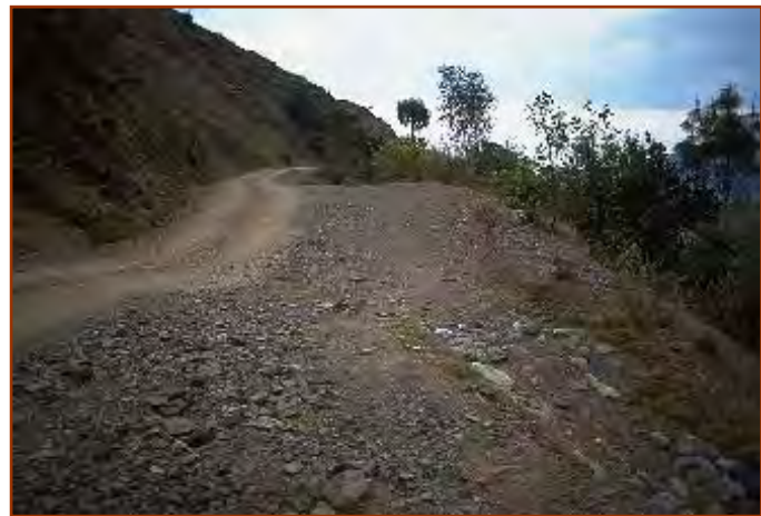
Low gradient roads with a competent rock surface can achieve sheet flow drainage with a 2% outslope.
