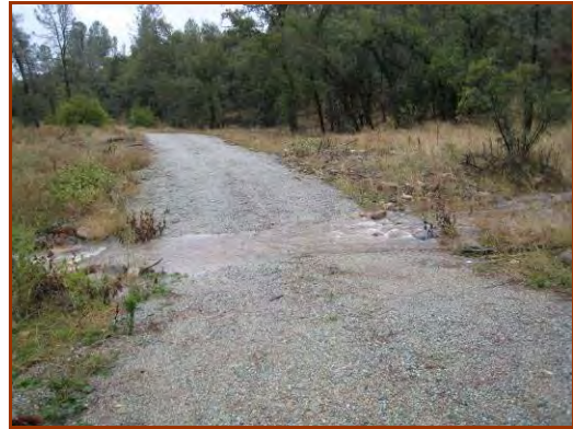
This ford or “armored dip” has a well-compacted structural sub-base (large cobbles) and then armored with stone. (J. McCullah photo, 2007)
