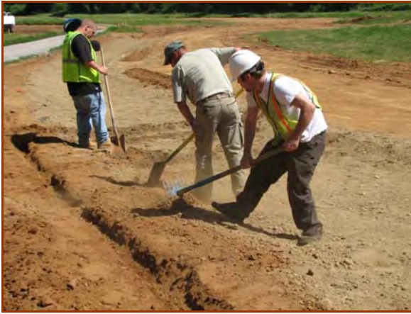
Longitudinal anchor trench should be 6 in wide x 6 in deep. On this test channel, the bottom was covered with 6 in of highly erosive decomposed granite soil (2 ft/s max permissible velocity).
