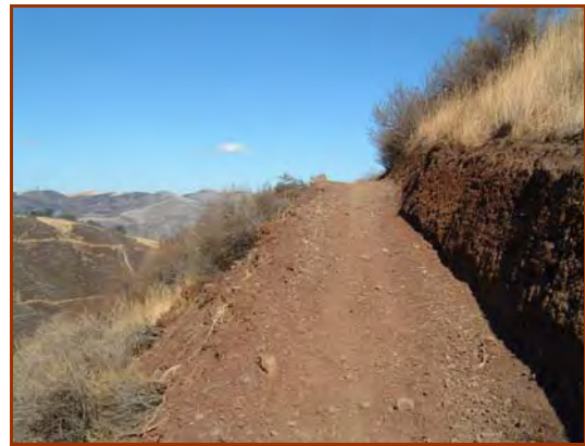
Construction of new SVRA trails should cause minimal disturbance by following natural land contours. (Carnegie SVRA)
