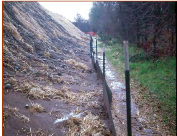
This huge stockpile was stabilized through the winter with straw mulch and silt fence installed by “slicing” with a silt fence machine (see PO-5 Stockpile Management).
