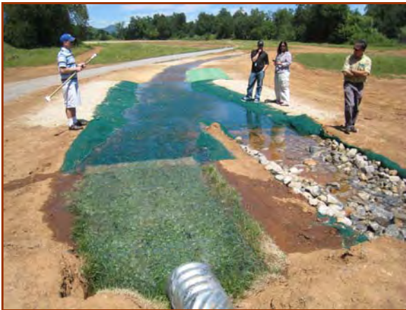
Observing the installed TRMs at the Shasta College ECTF by Caltrans Hydrologists, May 2007.
