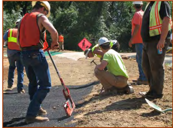
Follow the manufacturer's recommended anchoring pattern. The test site TRMs were anchored using hand driven anchor pins and a high speed stapler.
