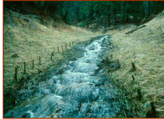
The soil-filled TRM (Enka Mat) protected the channel immediately. Reinforced with live staking. (J. McCullah, 1992)
