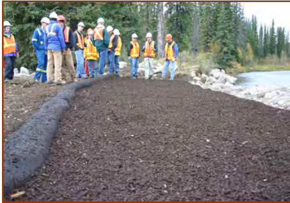
Two-inch thick compost blanket installed on Alberta DOT streambank project (at vane 1). Note compost sock installed for sediment control. (Canadian Rockies 2005)
