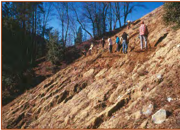
Brush Packing or Live Gully Fill Repair uses soil and sometimes straw/soil mix to fill the gully. (J. McCullah photo, 1992)
