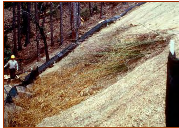
Live Gully Fill Repair relies on the use of willow branches (and sometimes geotextiles) to provide soil reinforcement. (J. McCullah photo, 1994)
