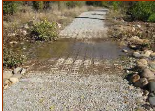
This low water crossing, designed for recreation and heavy equipment, is constructed from Articulated Concrete Blocks (ACBs). (J. McCullah photo, 2007)
