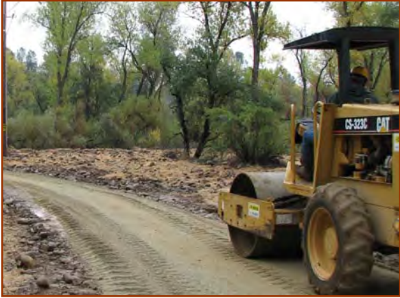
About every two years, base rock-surfaced roads should be ripped with a toothed grader and then re-graded, spread, moistened, and re-compacted.
