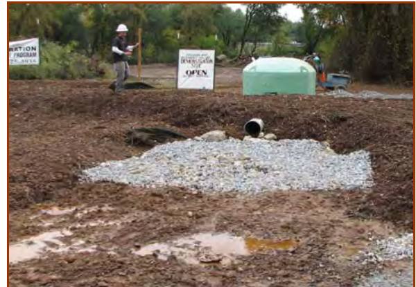
Apron is "overcut" to accommodate riprap thickness, and then lined with anchored geotextile.
