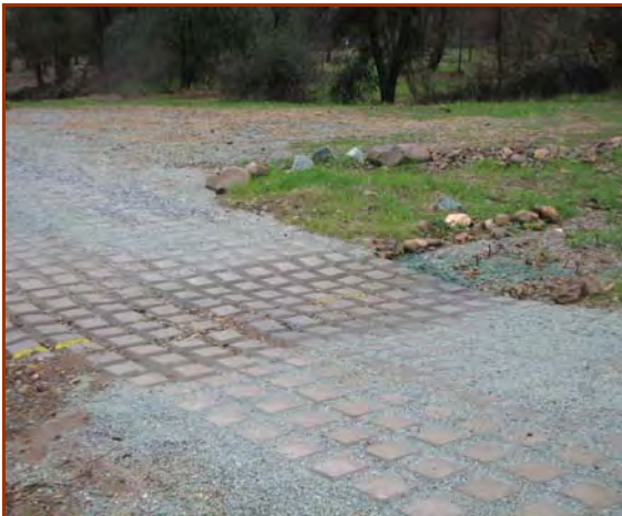
A cabled ACB after one year and several big storm flows in a watershed restoration project.
