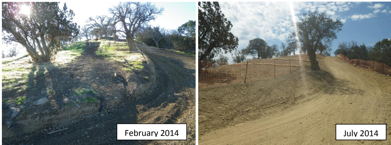
Figure 9. Rehabilitation Work in Knoll/Happiness. This shows an area of the Knoll that was closed to eliminate off-trail riding, recontoured, and wattled. Area will be hydroseeded before first rains.
