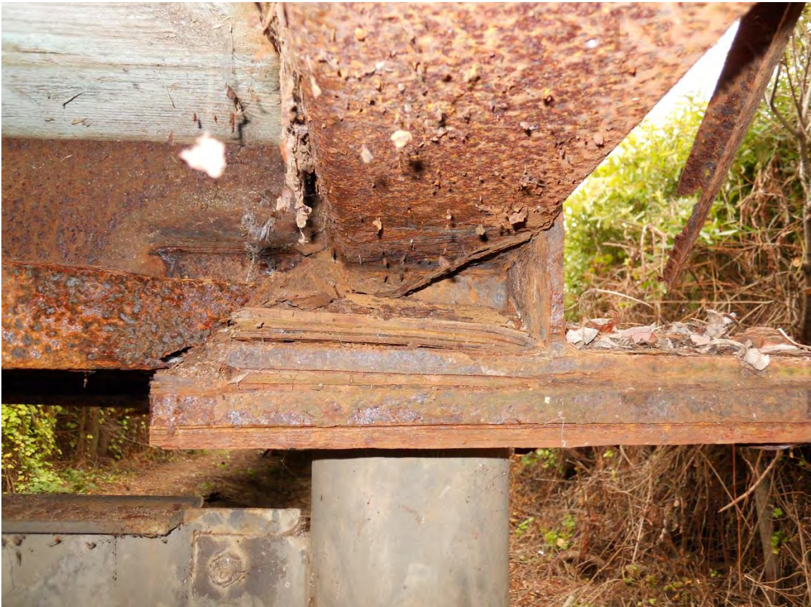
Bearing Plate Corrosion – Pier 2
