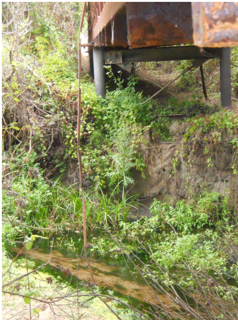
Stream Scour – Pier 3
