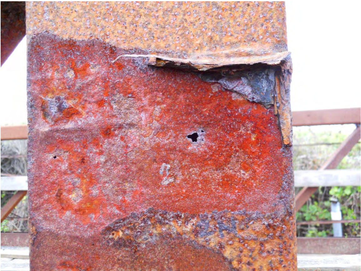
Truss Vertical at Guardrail Attachment [Section Compromised]
