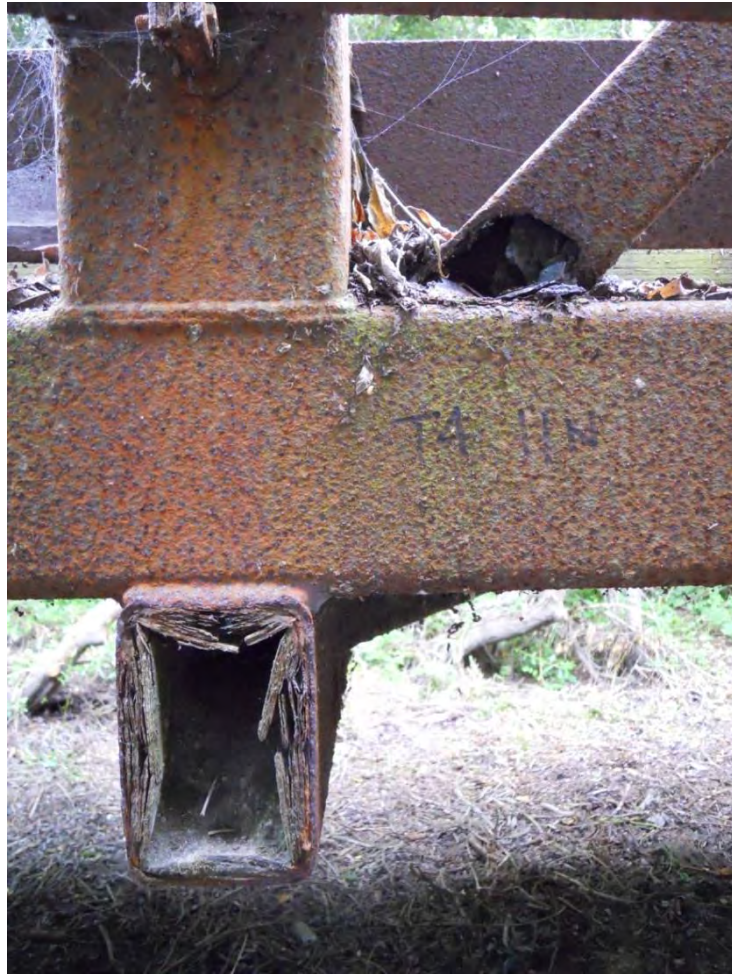
Typical Floor Beam and Brace Connection Corrosion – Span 4 [75% Loss of Section]
