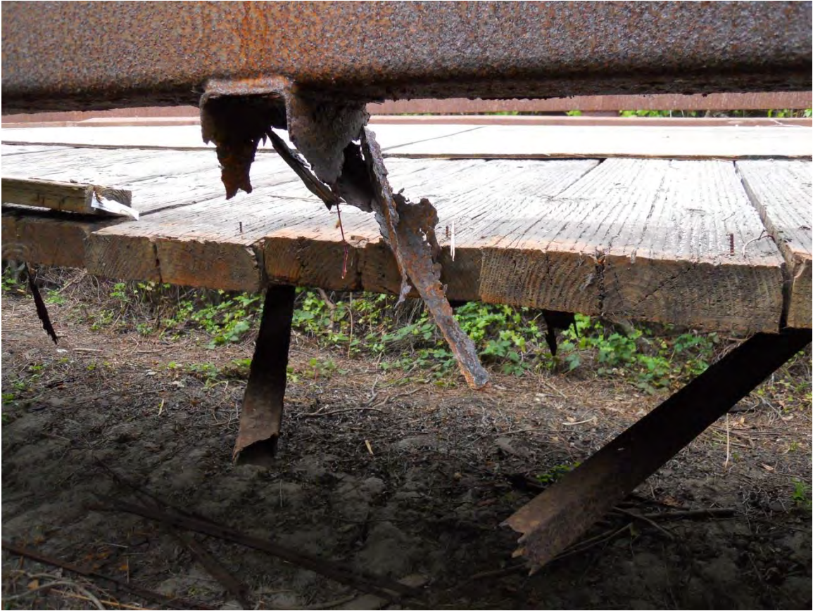
Collapsed Deck – Span 1
