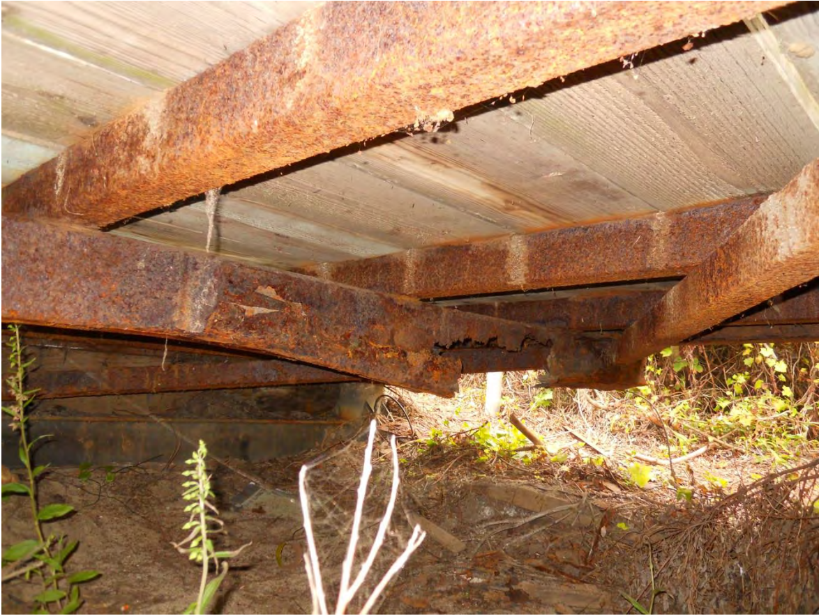
Floor Beam Corrosion Failure – Span 1, Panel 2
