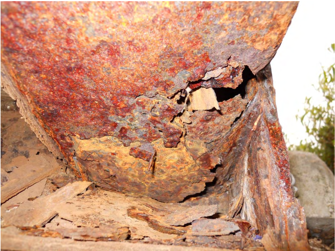
Bottom Chord Section Loss – Abutment 1
