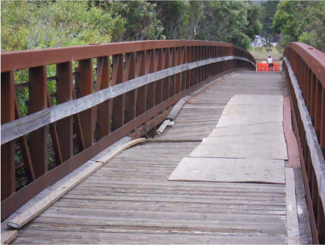
Collapsing Portion of Deck – Span 1 (Note Public Use)
