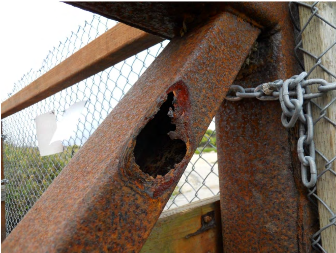
Truss End Diagonal Corrosion Hole – Span 1 [50% Loss of Section]
