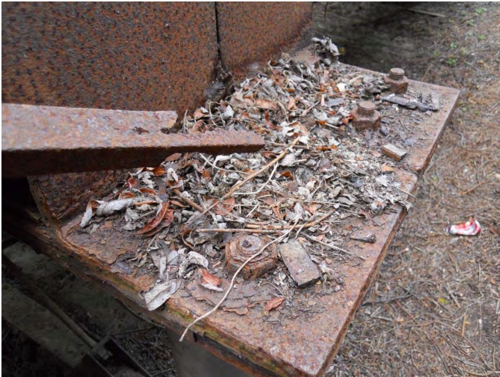
Bearing Plate Corrosion – Pier 3
