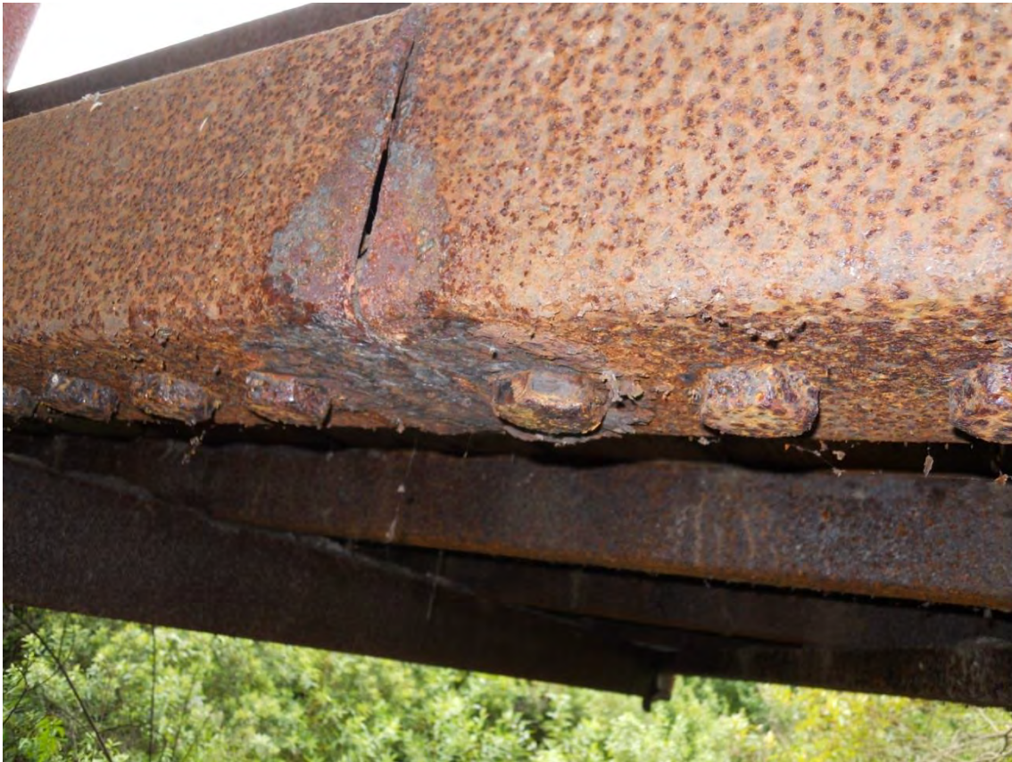
Bottom Chord Corrosion at Midspan Splice – Span 2 [50% Section Loss]
