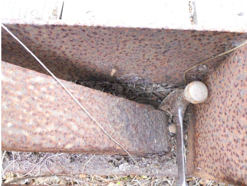
Truss Diagonal Section Loss at Connection to Bottom Chord at Deck Kick Plate – Span 4
