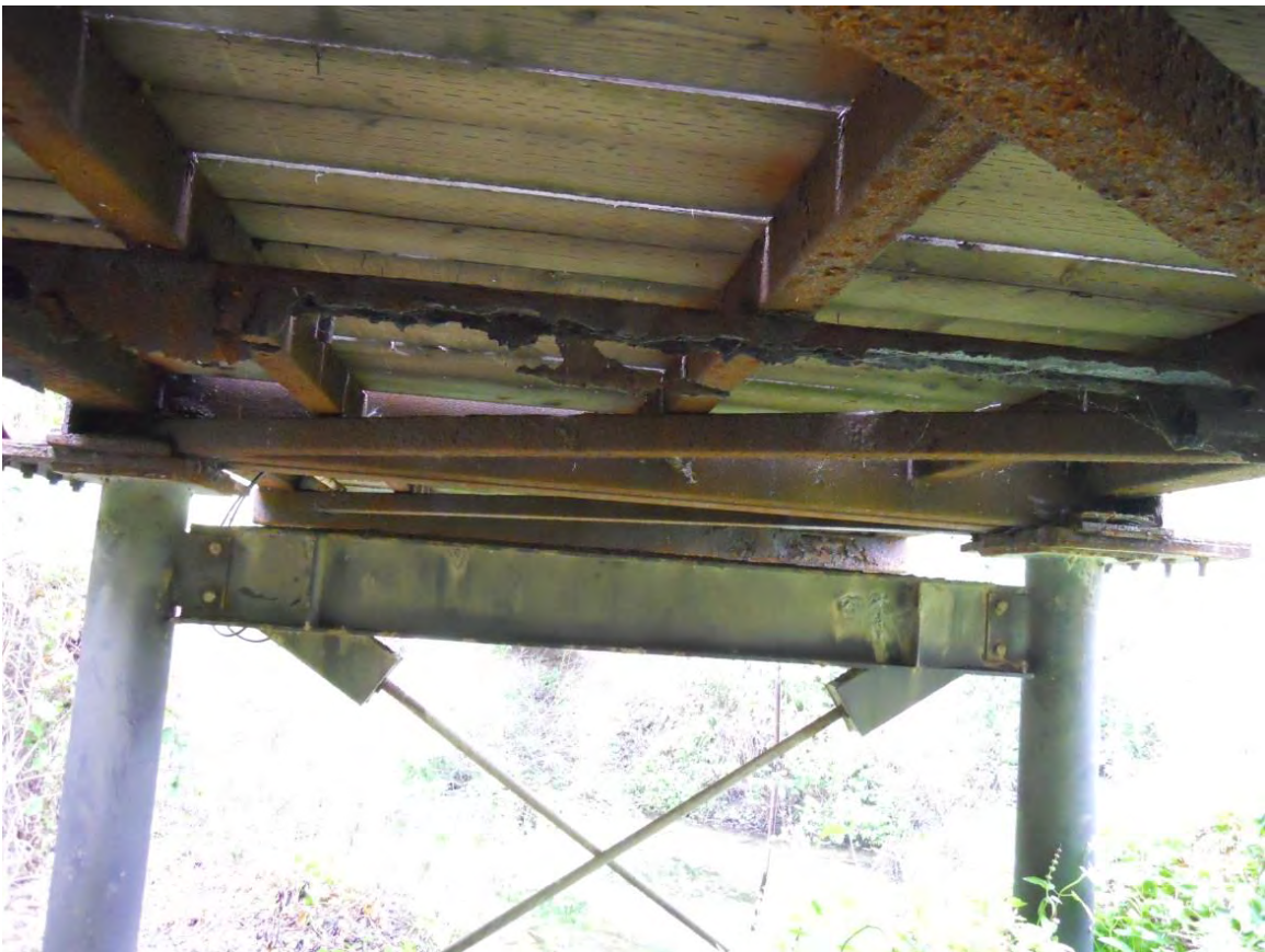
Floor Beam Corrosion – Pier 3 [100% Loss of Section]
