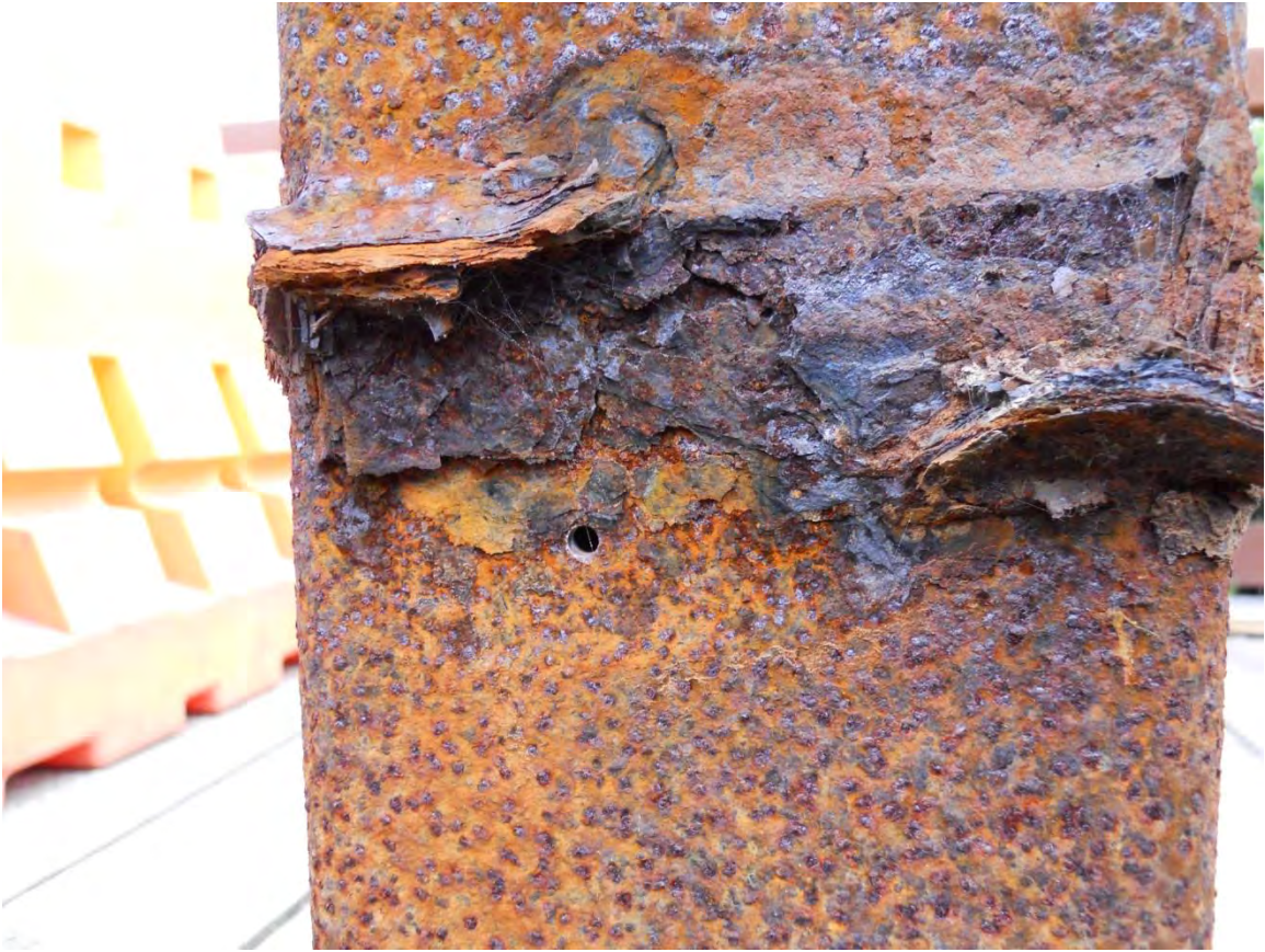
Truss Vertical – Span 1, Panel 3 [25% Loss of Section at Drilled Holes]
