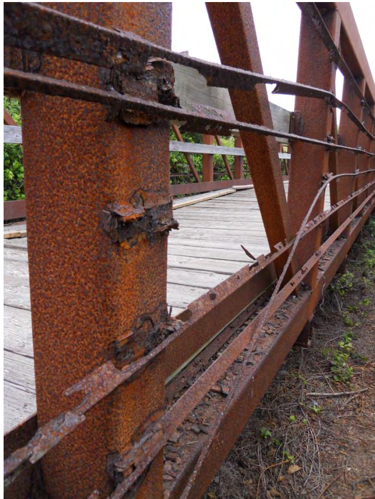
Typical Corrosion at Guardrail Runners
