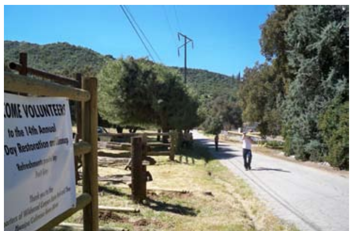
At Wildwood Canyon State Park, 400 feet of the planned 500 foot of lodge pole fencing was installed,
