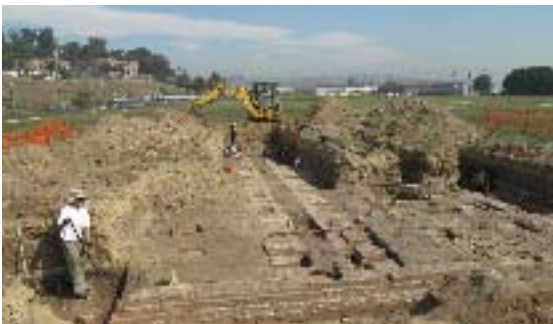
An exterior wall foundation of the Car Shop is seen in the foreground. Brendon Greenaway is excavating at the corner of the building in the foreground, while Barbara Tejada and Monica Aleman are excavating in the background and Dale Skinner is operating the backhoe.
