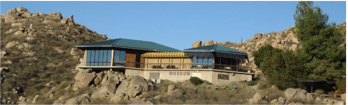
Top to Bottom: This “before” view of the visitor’s center shows a building in need of repair; the “after” view shows the new roof and ADA compliant doors.
