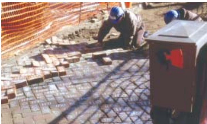
California Conservation Corpsmembers laying historic brick at Stanford Mansion State Historic Park
