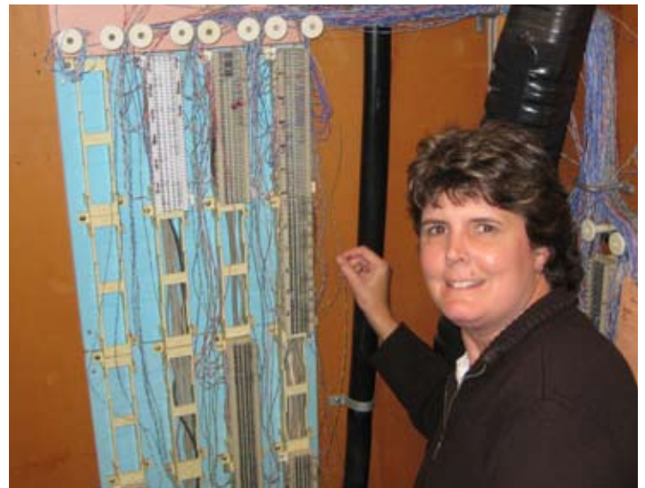
Tracy Hurtig poses with the inner workings of the headquarters phone lines.
