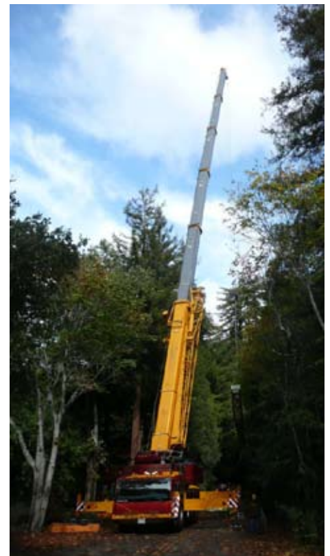
Crane used to lift and remove the bridge to the Big Sur campground
