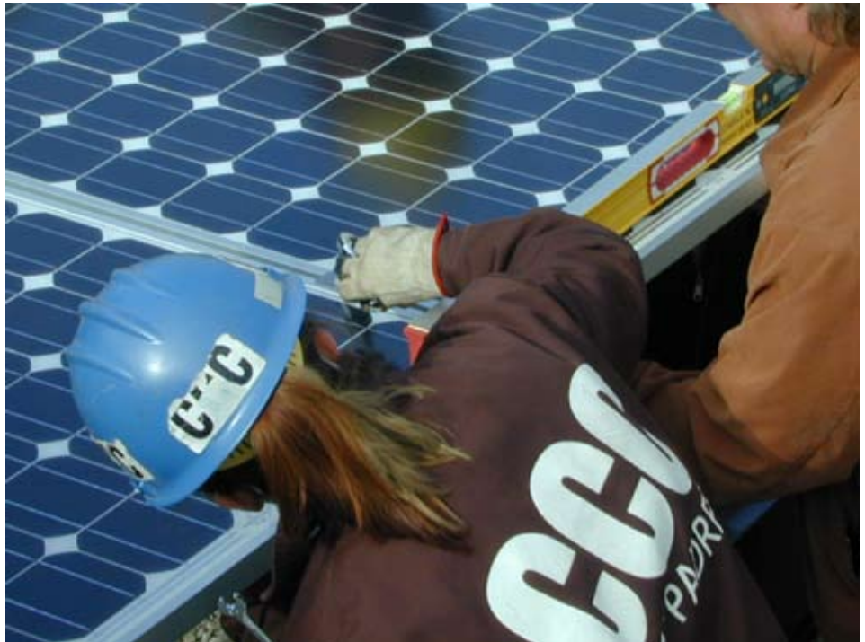
Members of the California Conservation Corps were essential to the installation of photovoltaic panels at Spooner’s Cove
