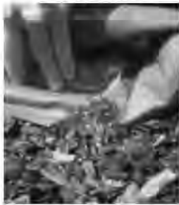
Clogged water release hole
