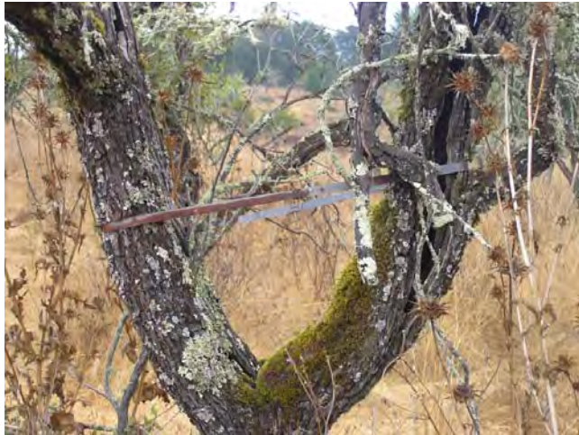
Figure 53: Contemporary photo of a metal brace installed to prevent scaffold limbs from splitting apart. The brace is approximately thirty years old ( NPS PWR, 2006 ).
