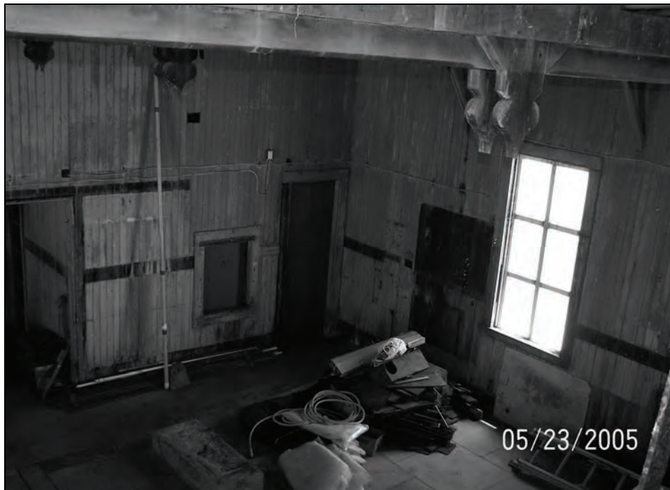
Figure 96. Interior of Fog Signal Building, 1899 Portion, 2005. Photograph shows door into Room 8. Note foundations for boilers and other equipment.
