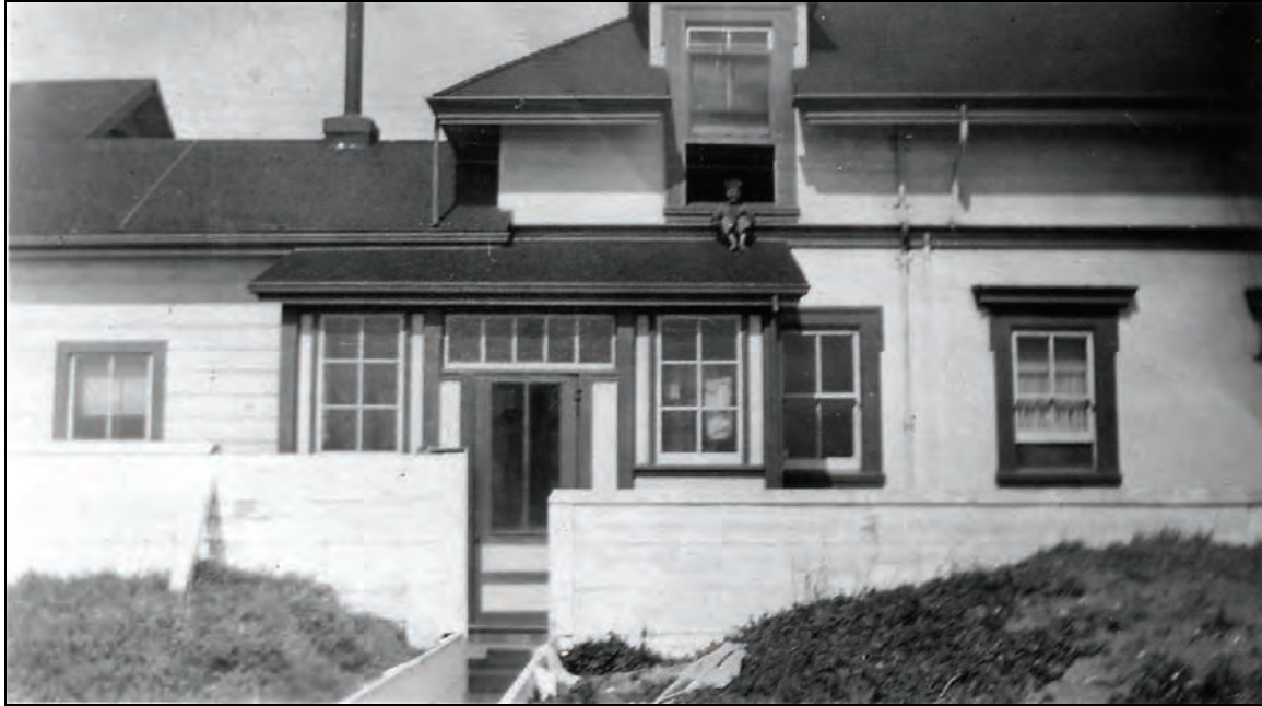
Figure 67. Rear (west) of Keeper's Dwelling (1906 Addition), showing Separation between Original Building (on left) and Addition on Right, 1926.
