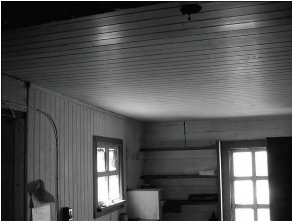
Figure 94. Interior of 1881 Section of Fog Signal Building, West Corner, 2005. Note tongue and groove siding on wall to left and ceiling sheathing, and shiplap sheathing on wall at right.
