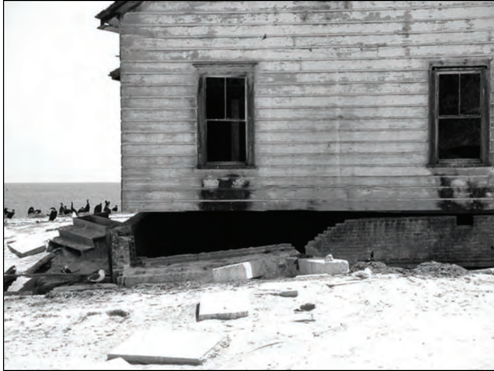
Figure 65. Keeper's Dwelling, Original Portion, showing Brick Foundation and Deterioration to North Corner, 2005.
