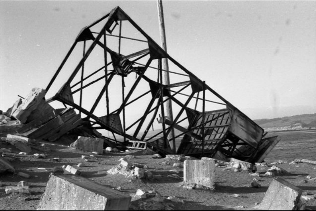
Figure 82. Steel light tower following dismantling by state, 1982. Catalog #24754 Catalog #24743, California State Parks, Archaeology Laboratory, West Sacramento.
