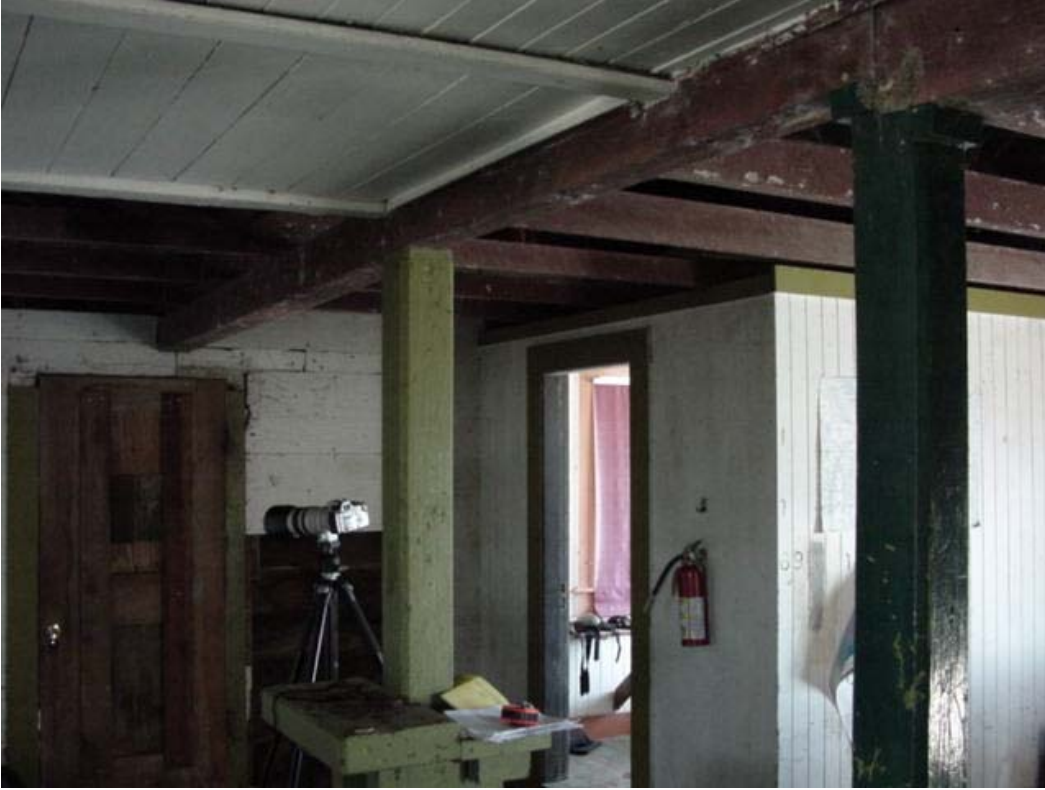
Figure 72. Interior of 1881 section of fog signal building, east corner, showing Room 2 and posts supporting beam, 2005
