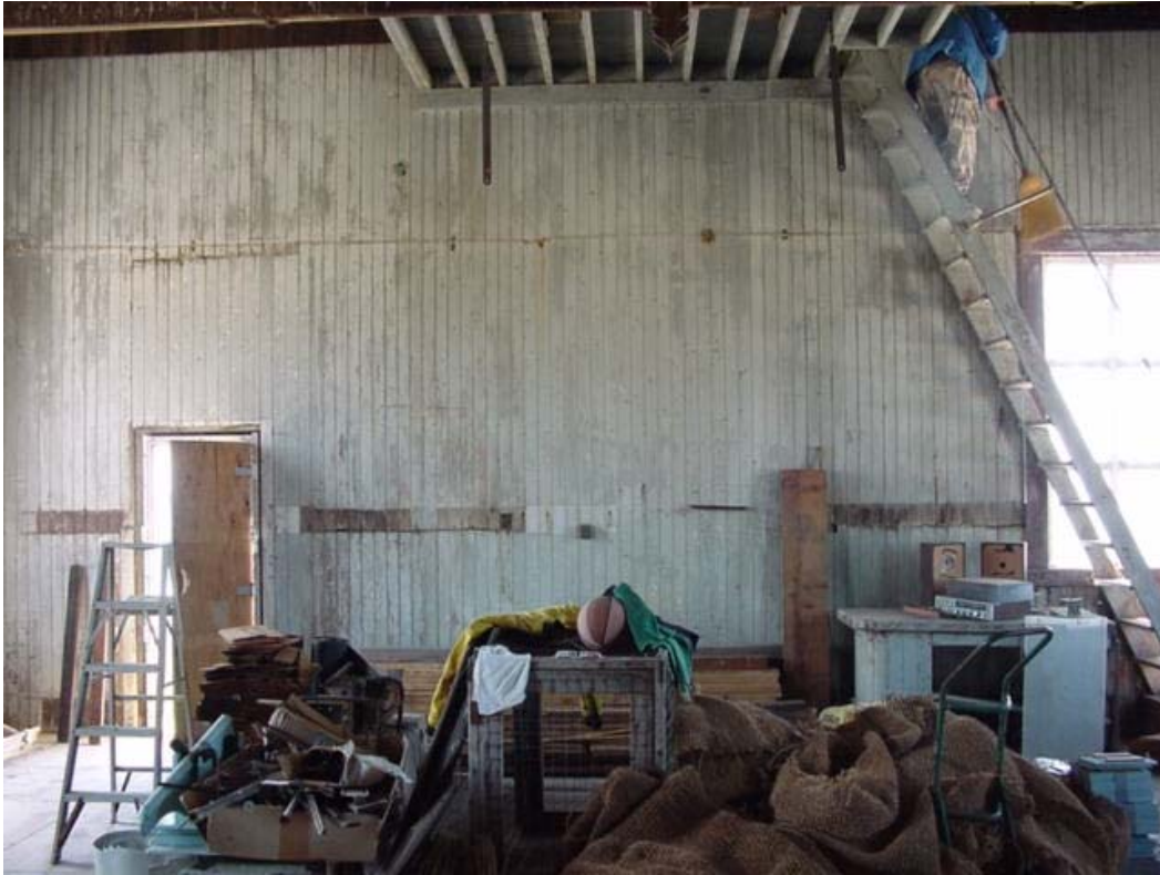
Figure 74. Interior of 1899 fog signal building, southwest wall, 2005. Loft visible at top of photograph was original location of fog signal whistles.
