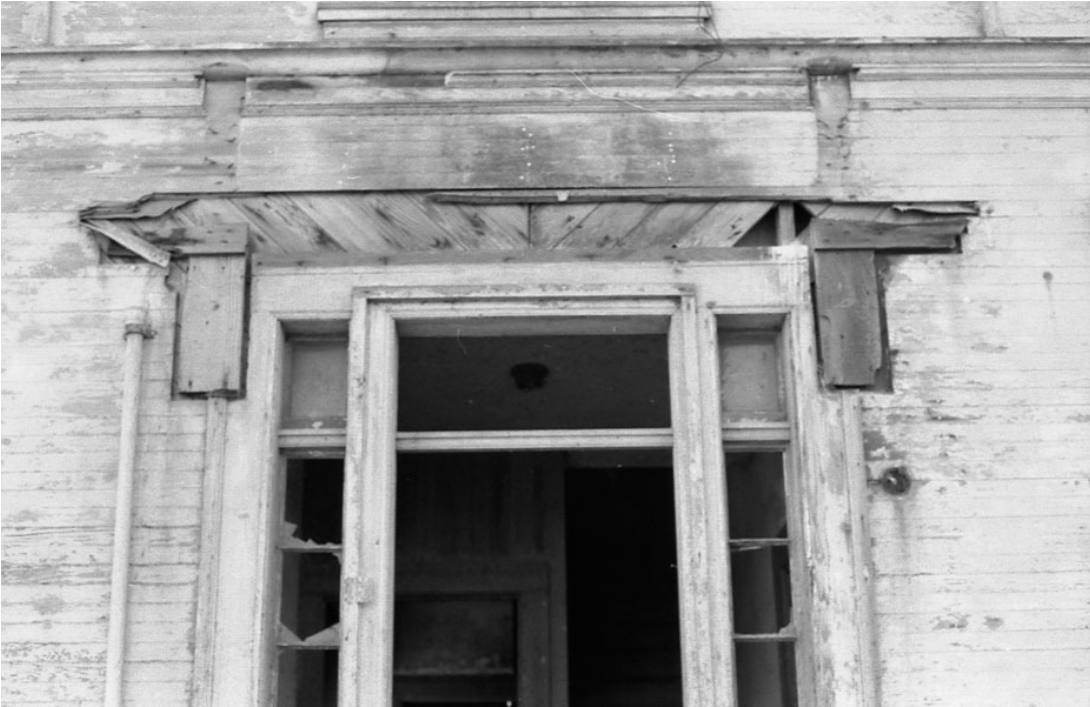
Figure 50. Front (east) entrance to keeper's dwelling (1906 addition), 1982. Note scar from portico and boarded transom. Catalog #24740, California State Parks, Archaeology Laboratory, West Sacramento.
