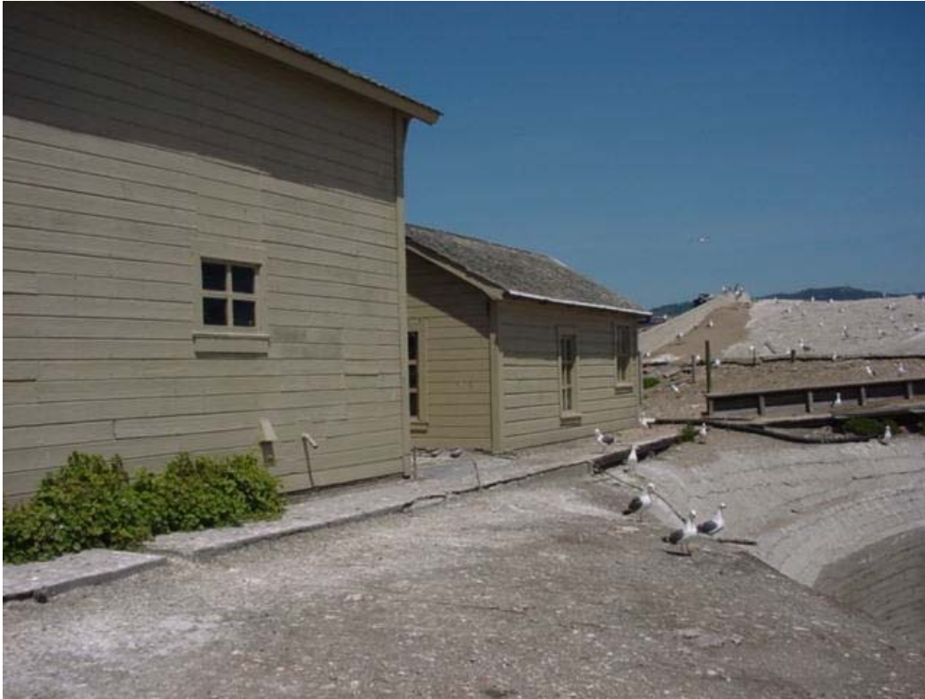
Figure 70. Fog signal building looking north, 2005. Note concrete retaining wall at right, and remains of wood walkway.
