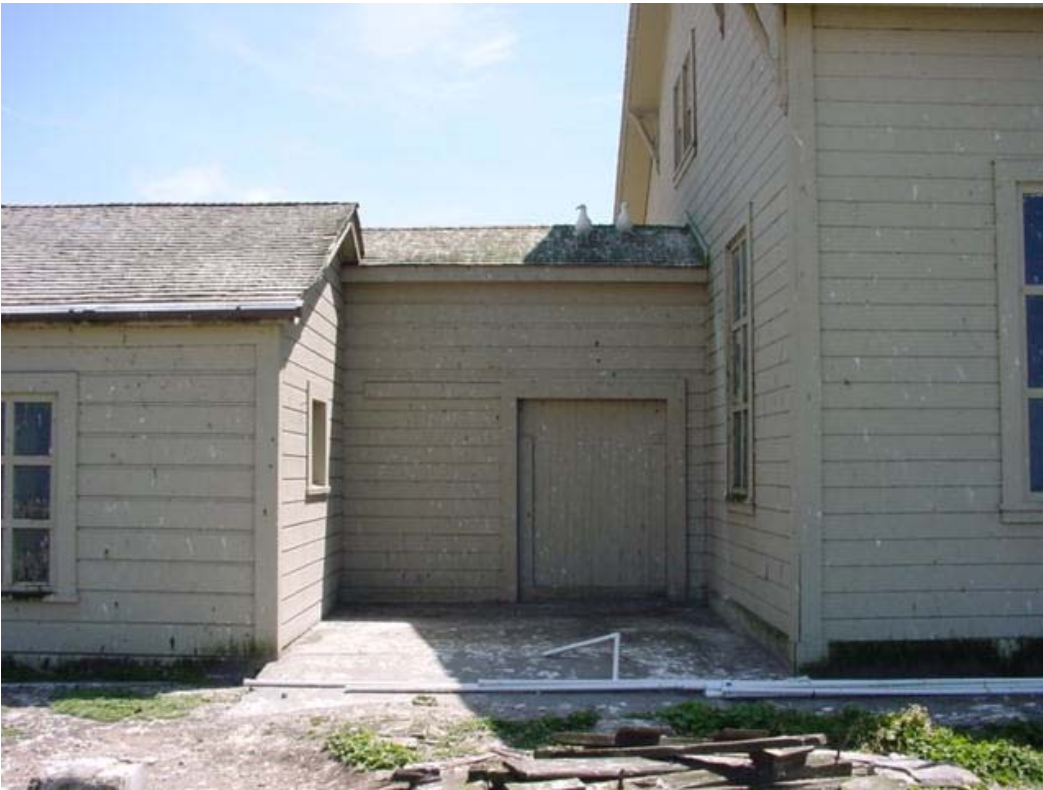
Figure 68. Fog signal building: gallery connecting 1881 portion at left and newer (1899) building at right, 2005.
