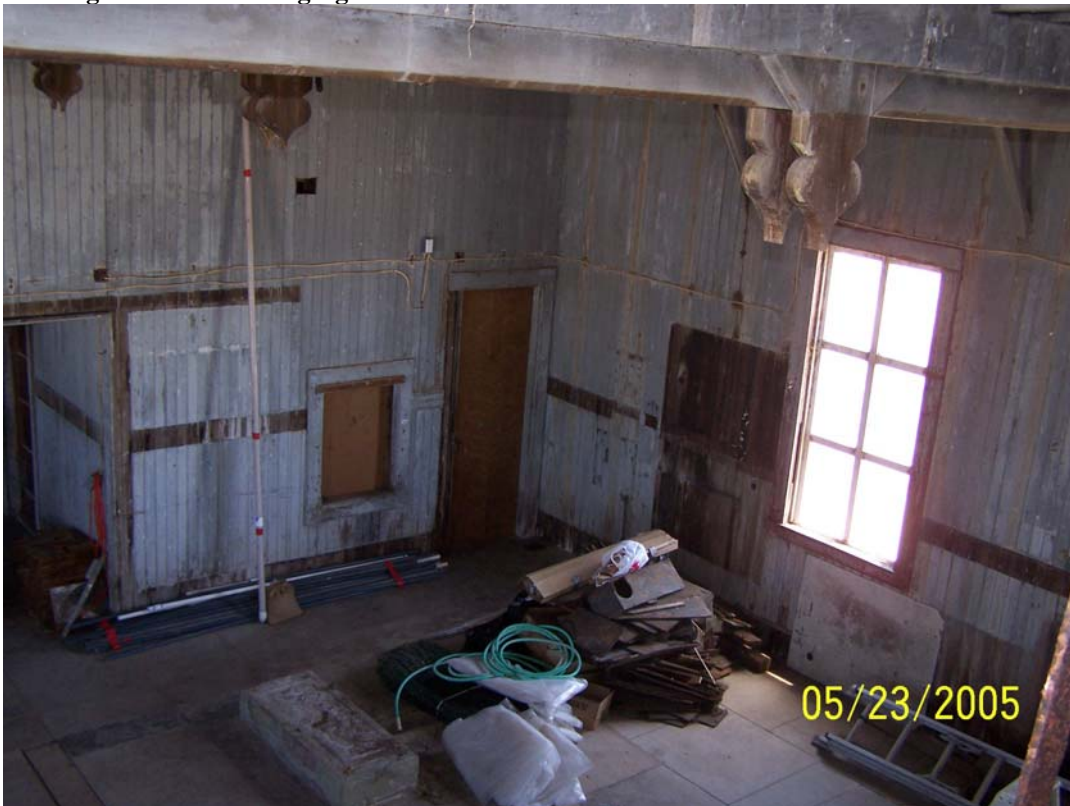
Figure 75. Interior of fog signal building, 1899 portion, showing door into Room 8, 2005. Note foundations for boilers and other equipment.
