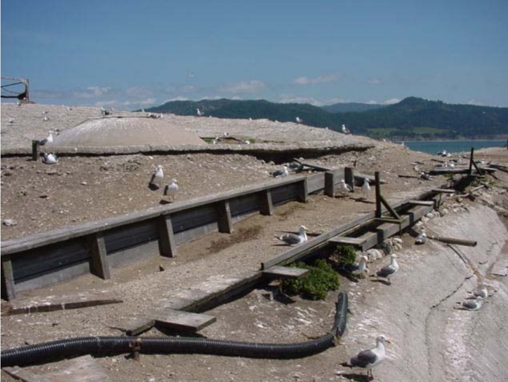
Figure 103. Remains of wood walkway connecting keeper's dwelling with fog signal building, 2005.
