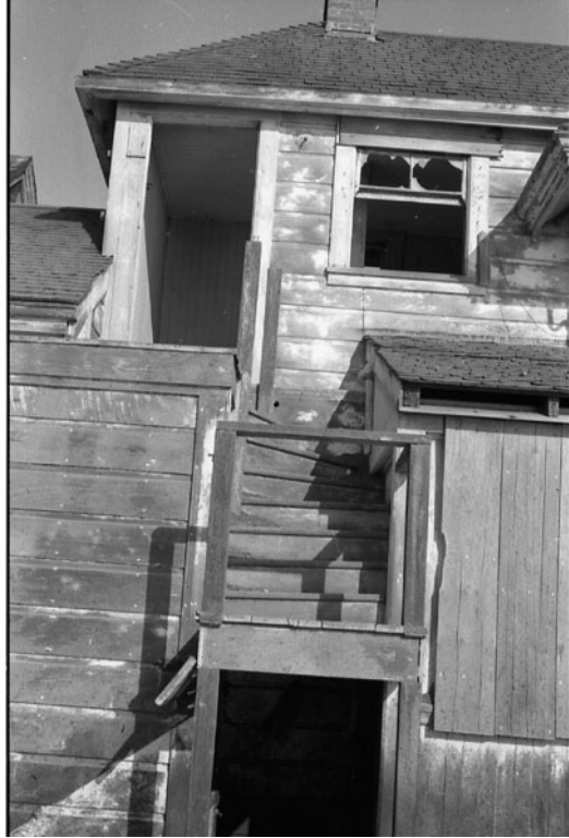
Figure 48. Rear of Keeper's dwelling (1906 addition), stairway to landing, west side, 1982. This stairway was added sometime later judging by previous figure. Catalog #24738, California State Parks, Archaeology Laboratory, West Sacramento.
