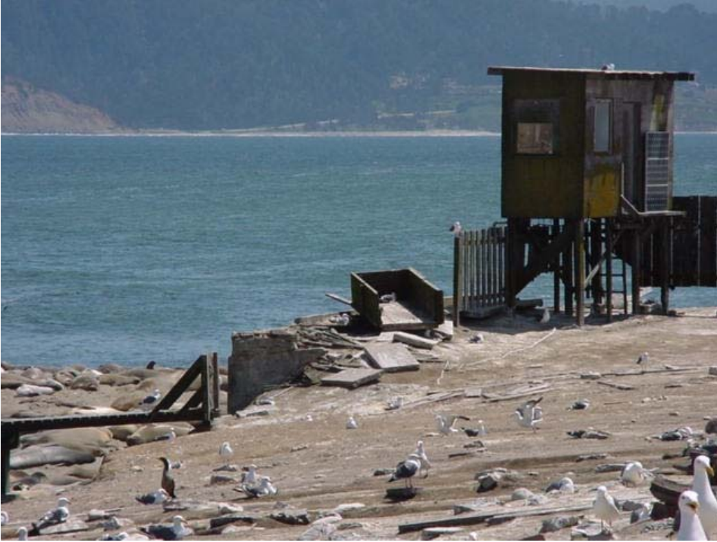
Figure 95. Foundation of boathouse to left of modern blind, 2005. Pier is visible at left.
