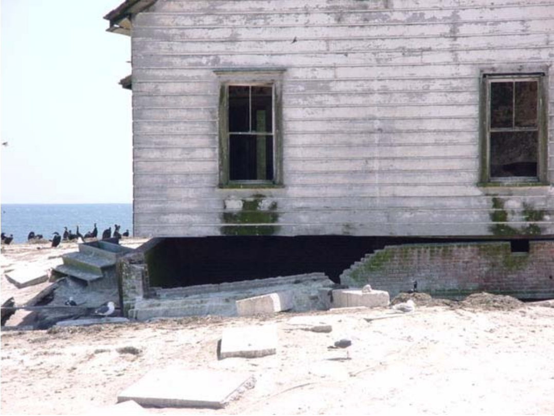
Figure 43. Keeper's dwelling, original portion, showing brick foundation and deterioration to north corner, 2005.
