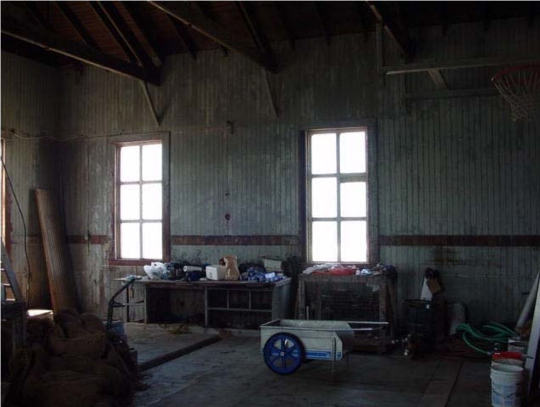
Figure 76. Interior of 1899 fog signal building, northwest wall, 2005. Note tongue and groove sheathing, and lower portions of roof trusses.
