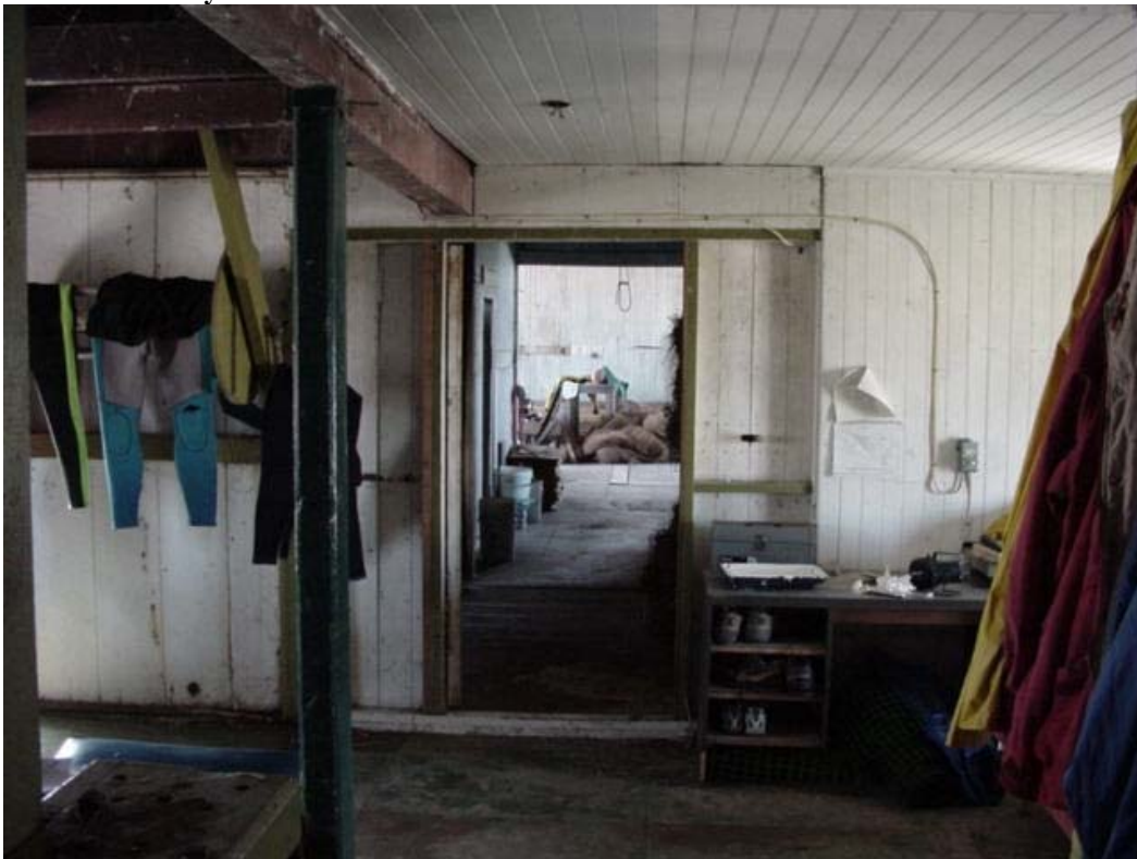
Figure 71. Interior of 1881 section of fog signal building looking through gallery (southwest) to 1899 building, 2005.
