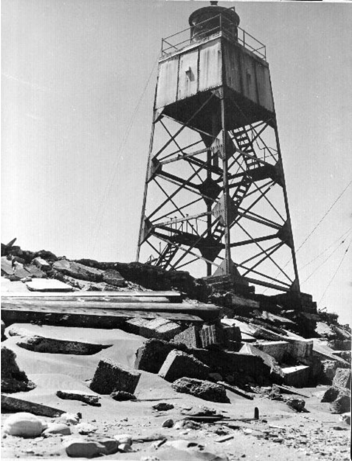
Figure 79. Steel light tower, ca. late 1950s. U.S. Coast Guard photograph, California State Parks.
