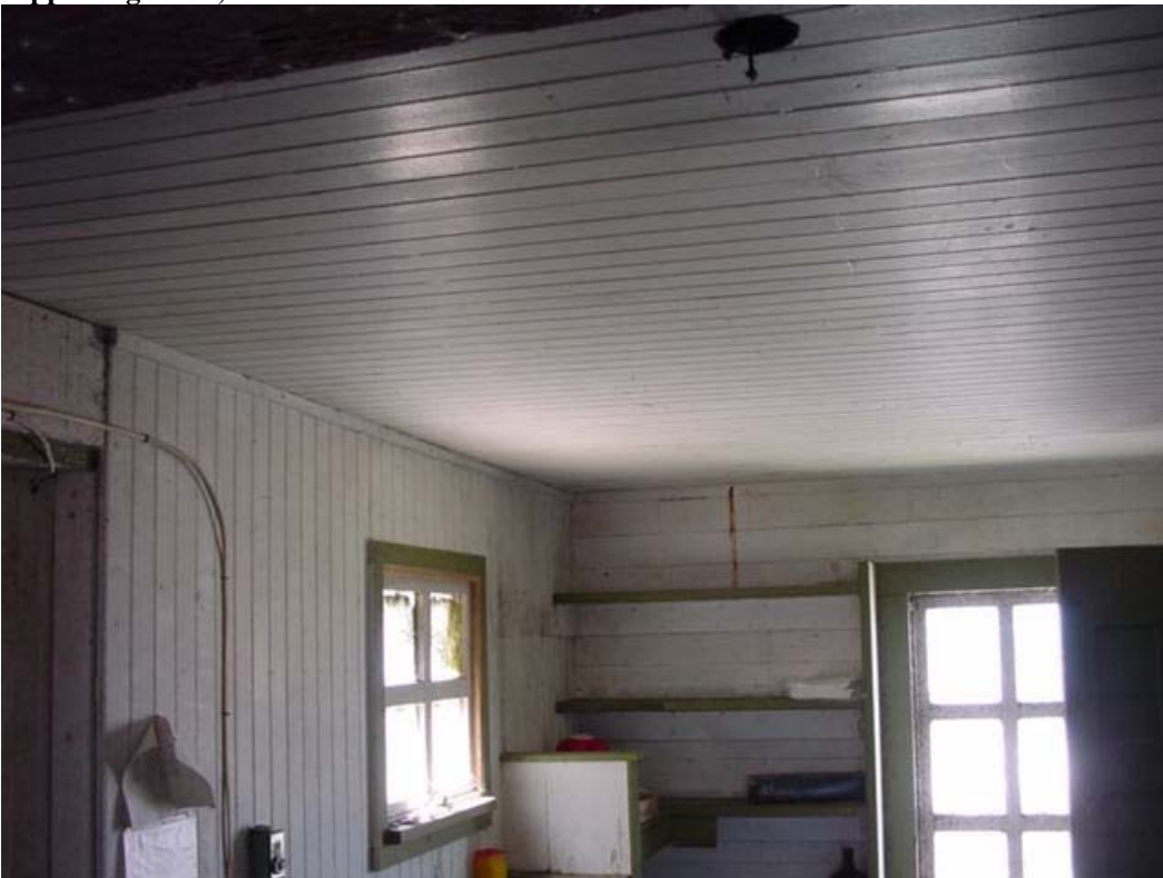
Figure 73. Interior of 1881 section of fog signal building, west corner, 2005. Note tongue and groove siding on wall to left and ceiling sheathing, and shiplap sheathing on wall at right.
