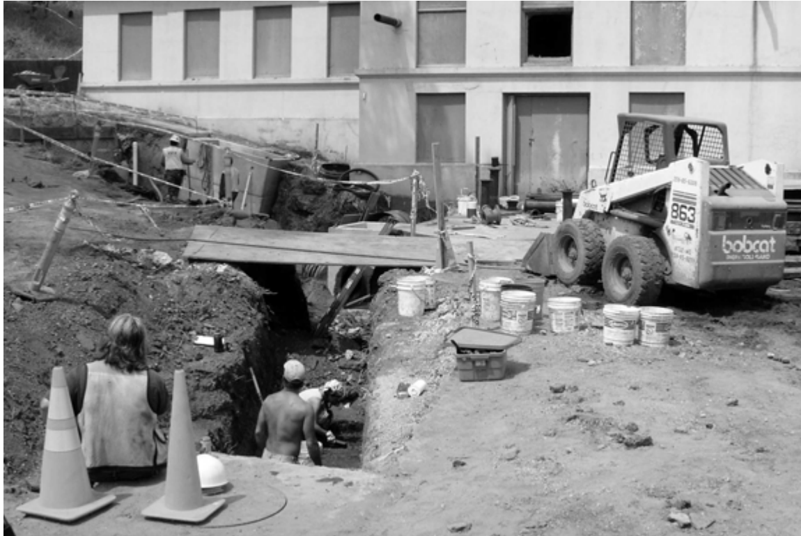
Figure 14. Storm Drain Trench in Front of Central Heating Plant, Locus B, Trench 15.
