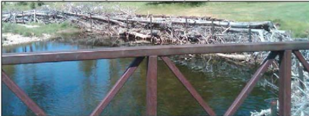
An undersized bridge on Hole 6 – the par 3. The logs placed horizontally are band-aids aimed at stopping the severe cut-bank erosion just downstream from the bridge. Just upstream from the bridge has been incised by the narrowing of the river.
