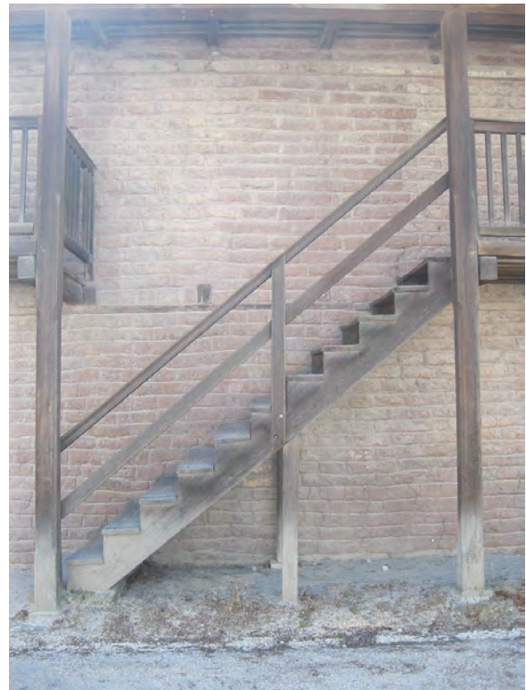
Figure A73. Detail of one of two stairs to the second floor balcony. Note the staining on the columns from water backsplashing
