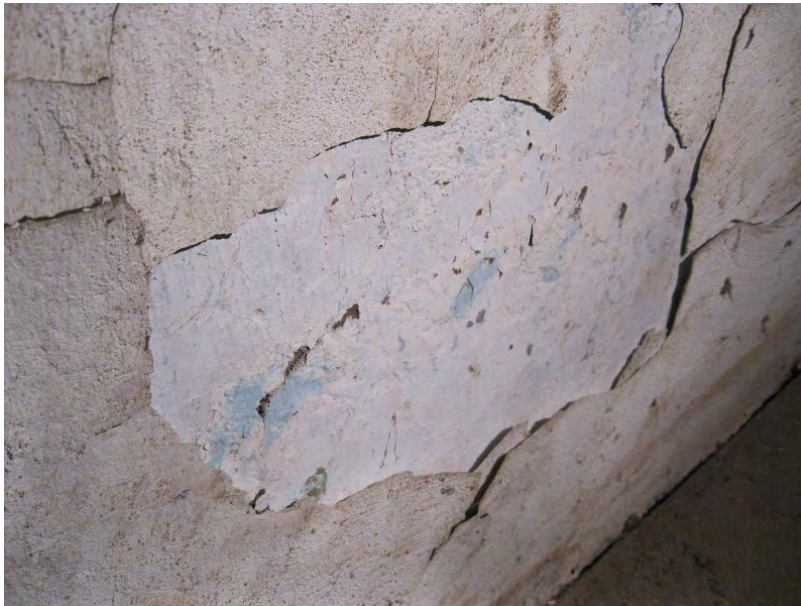
Figure 25. There are several layers of plaster and paint finishes on the second floor of the Servants' Quarters. This image shows the complicated stratigraphy found in areas of current damage.
