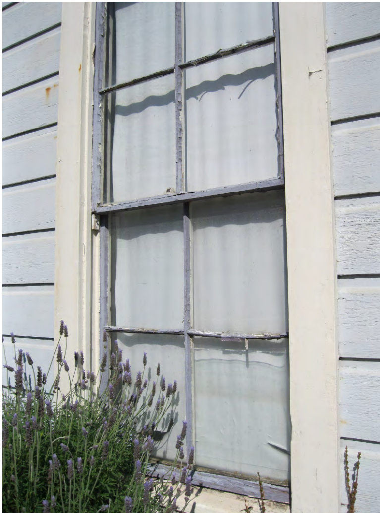
Figure 40. Windows on the west elevation of the Hotel Annex all exhibit dry and cracked glazing putty, failing paint finishes, and warping sash elements. The muntins are very thin, making them more susceptible to weathering than more contemporary designs (photo: Garavaglia Architecture, Inc., April 2013).
