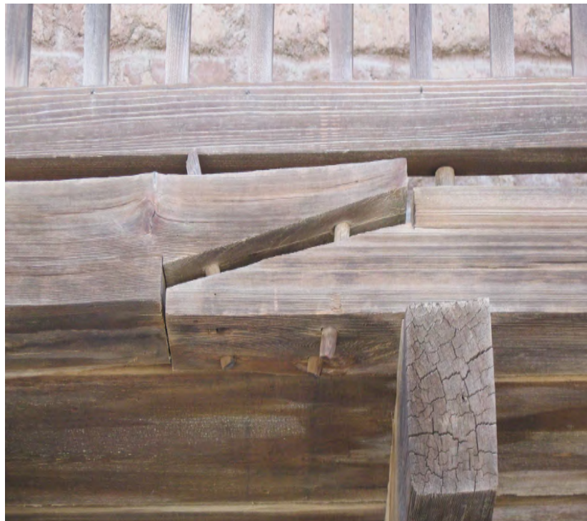
Figure 45. The exterior hallway on the east elevation of the Servants' Quarters is a contemporary version of an original feature. It was rebuilt using a combination of modern and traditional techniques. Here, an area of wood dowel pinning is starting to loosen and requires immediate attention (photo: Garavaglia Architecture, Inc., April 2013).
