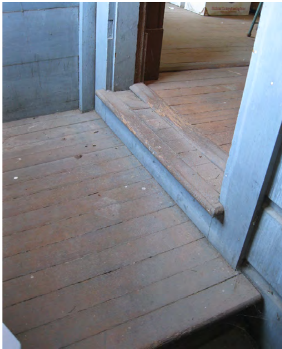
Figure A36. Landing at the top of the external stair to the second floor.
