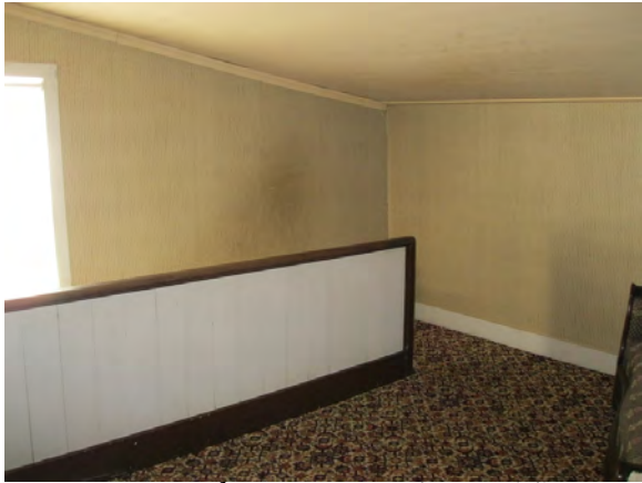
Figure A20. Northwest corner of second floor. This area was converted to a bathroom c.1914. The bathroom was removed in the 1960s.
