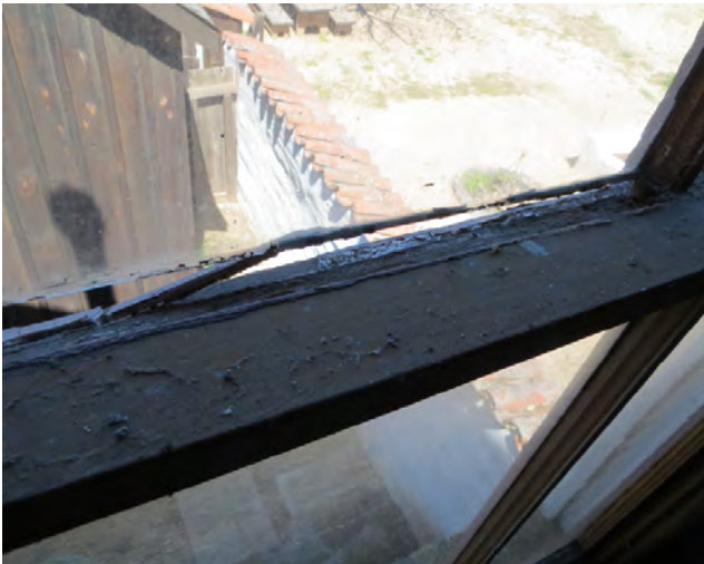
Figure 34. Window damage is especially severe on the second floor of the Kitchen Annex. This image shows deteriorated glazing putty, missing muntin elements, and loose glass (photo: Garavaglia Architecture, Inc., April 2013).
