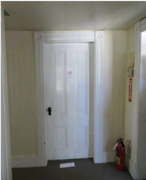
Figure A48. Door to the kitchen with original wall finishes and modern drop ceiling.
