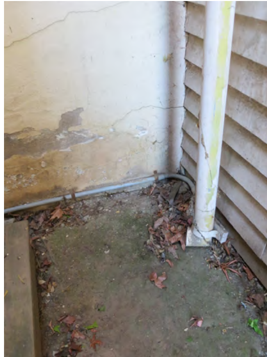
Figure 30. Downspouts on the rear elevation of the Toscano Hotel deposit rainwater at grade, directly adjacent to the building foundation. This downspout is at the northeast corner of the building (photo: Garavaglia Architecture, Inc., April 2013).
