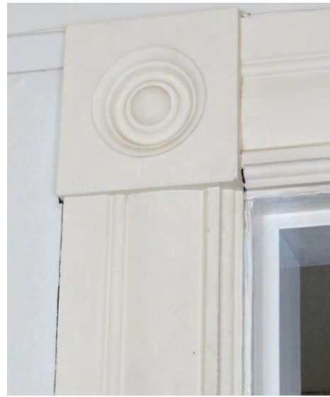
Figure 38. Contemporary finishes have been applied over original finishes throughout the Hotel Annex. Here, 1/4" fiberboard has been installed over the original plaster walls. As a result, the original bulls-eye trim is flush with the wall surface (photo: Garavaglia Architecture, Inc., April 2013).
