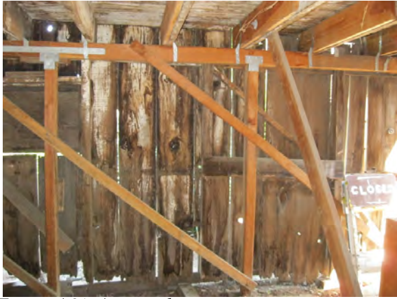
Figure A91. A secondary support structure was installed to prevent the barn from collapsing.
