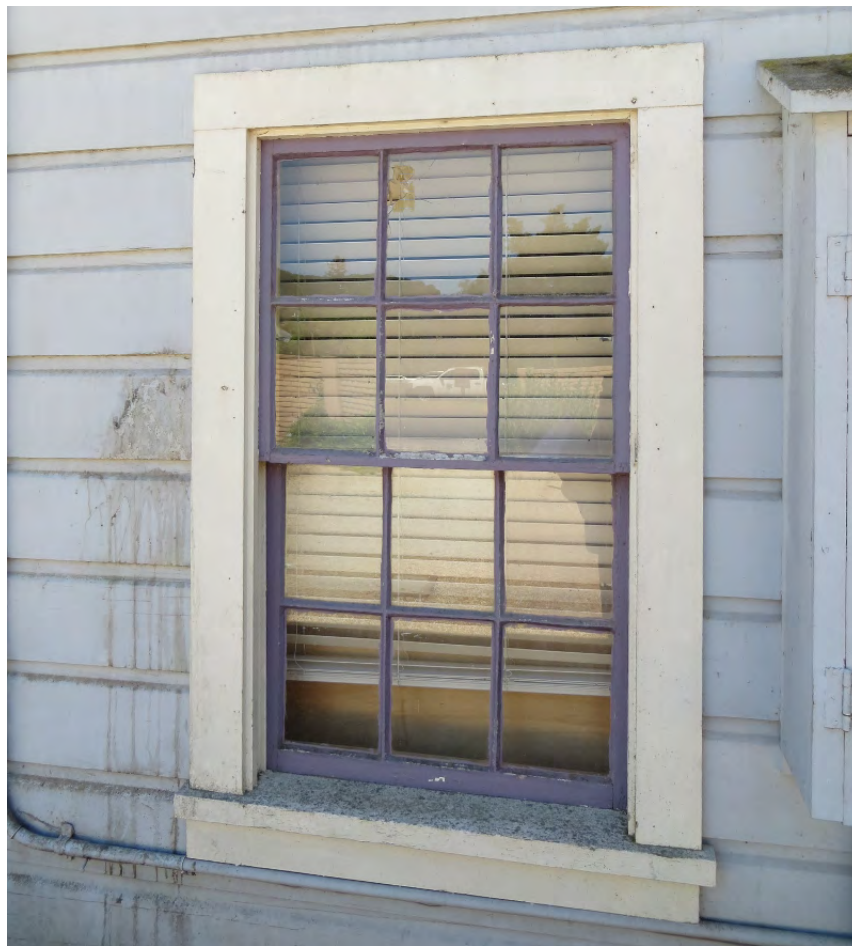
Figure 43. The first floor window on the Tank House faces north. It is fairly protected from harsh sun and winds, but still shows signs of paint failure and cracked putty (photo: Garavaglia Architecture, Inc., April 2013).
