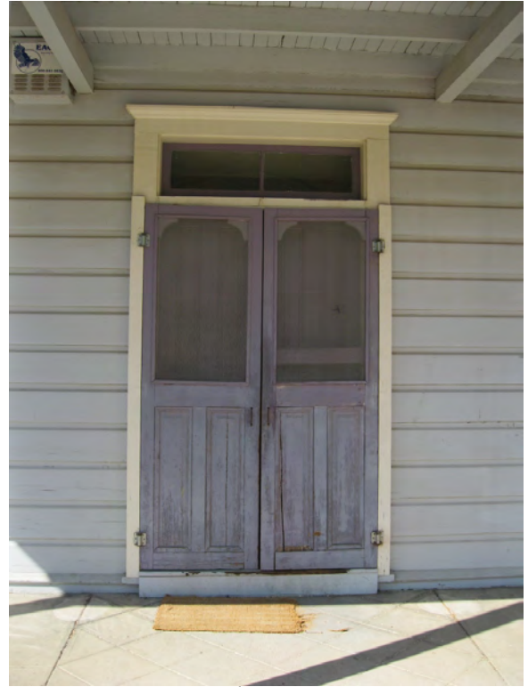
Figure A45. Detail of the front screen doors. There is damage to the eastern door.
