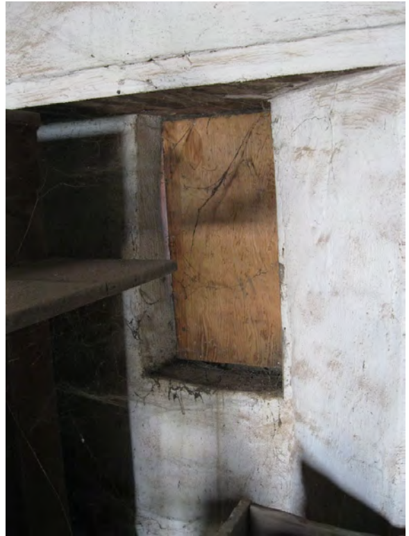
Figure A83. A first floor opening has been boarded up.
