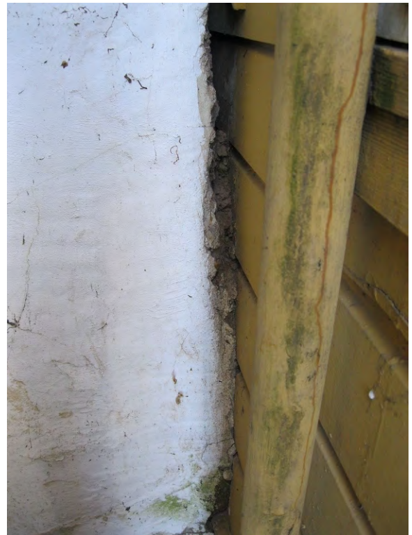
Figure A27. Detail the east elevation where it touches the older adobe Barracks building.
