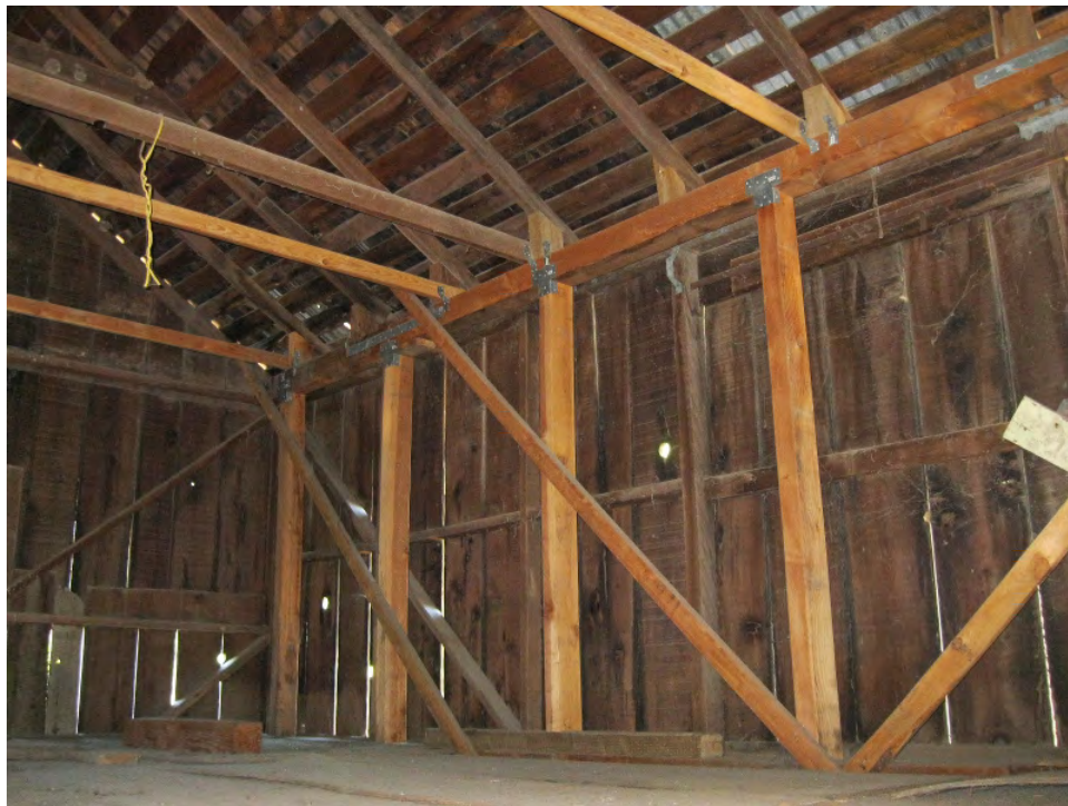
Figure 26. A secondary support frame has been installed in the barns to prevent them from collapse (photo: Garavaglia Architecture, Inc., April 2013).
