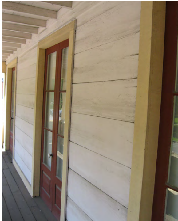
Figure A8. The siding under the porch on the second floor appears to be original. Note the large width of the siding boards.
