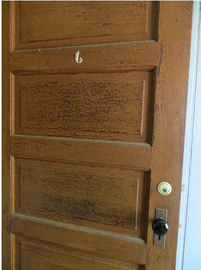
Figure 36. The door finishes on the second floor of the Kitchen Annex are failing. The surface coating has shrunk and bubbled on the exterior face of the doors. In general, the interior faces are less damaged (photo: Garavaglia Architecture, Inc., April 2013).
