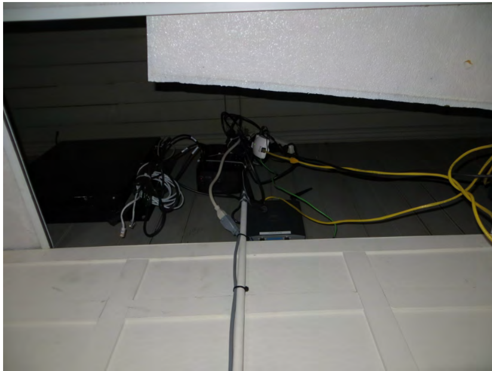
Figure 24. Drop ceilings and other contemporary finishes obscure the original architectural details in many rooms in the Hotel Annex (photo: Garavaglia Architecture, Inc., April 2013).
