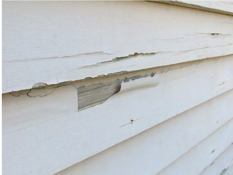
Figure 27. Typical finish failure on the Toscano Hotel. It is worst on the west side of the building (photo: Garavaglia Architecture, Inc., April 2013).
