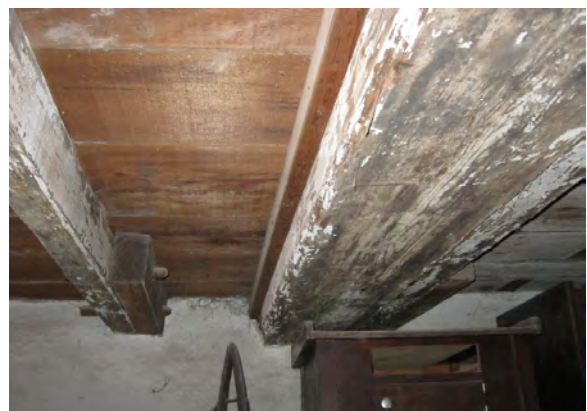
Figure A77. Note the width of the beam to the right.
