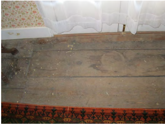
Figure A17. Water is damaging the floorboards on the second floor. These boards may be original.
