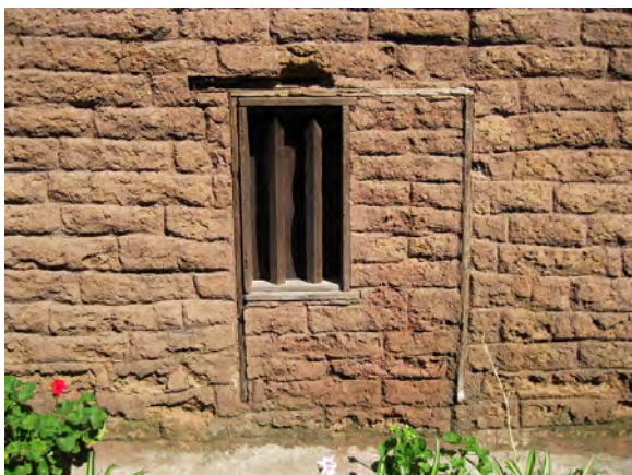
Figure A68. Detail of a former window or door that has been filled in on the west elevation.
