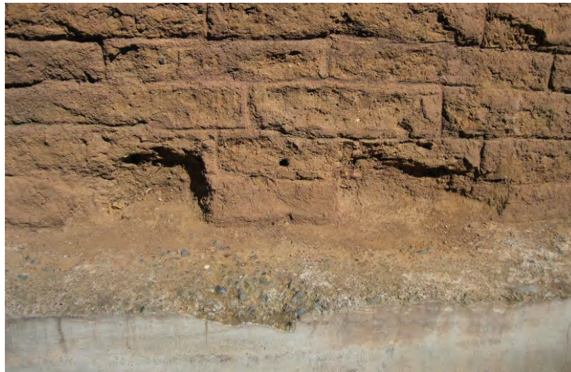
Figure 44. The concrete curb on the west side of the Servants' Quarters may be trapping moisture and forcing it to migrate further up the wall. As it evaporates, it can spall the fragile adobe surface (photo: Garavaglia Architecture, Inc., April 2013).
