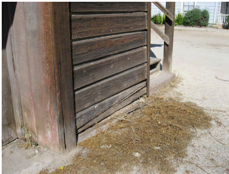
Figure 48. As the birds are nesting, they are pushing building materials out through gaps in the wood boards. Here straw from the adobe insulating fill has been deposited at the base of the wall (photo: Garavaglia Architecture, Inc., April 2013).
