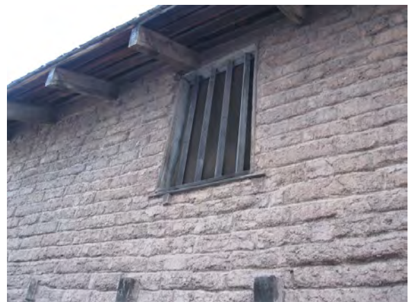
Figure A69. Second floor window opening with a wooden grate.
