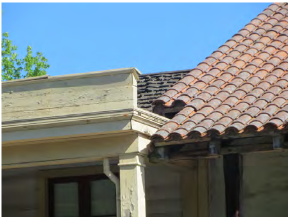
Figure A5. Overlapping roof structure of the Barracks Building and the Toscano Hotel porch.
