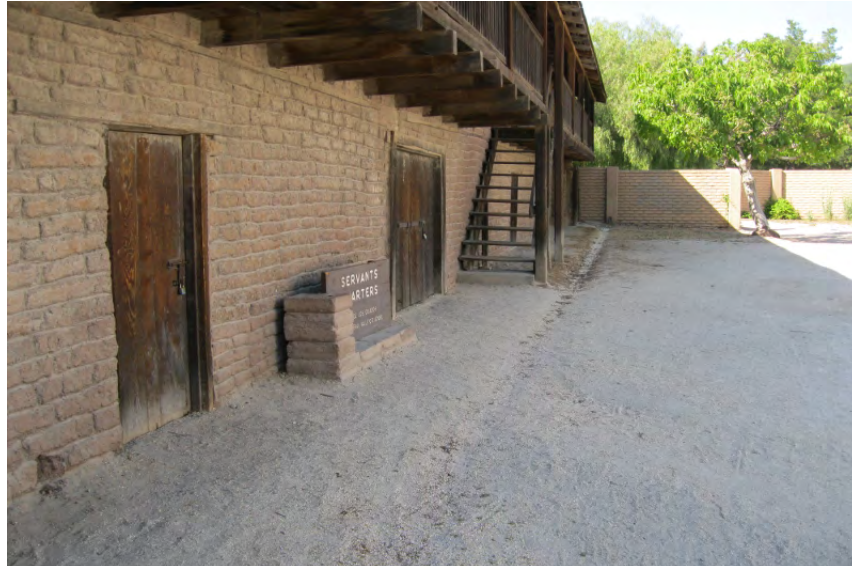
Figure 52. The lack of gutters on the Servants' Quarters allows water to drain directly off the roof and into the courtyard. A shallow indentation under the eave has resulted. Combined with poor grading, some water is draining to the building instead of out into the courtyard (photo: Garavaglia Architecture, Inc., April 2013).
