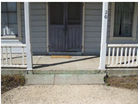
Figure A42. Detail of the green concrete front porch deck. The step does not comply with current accessibility requirements.
