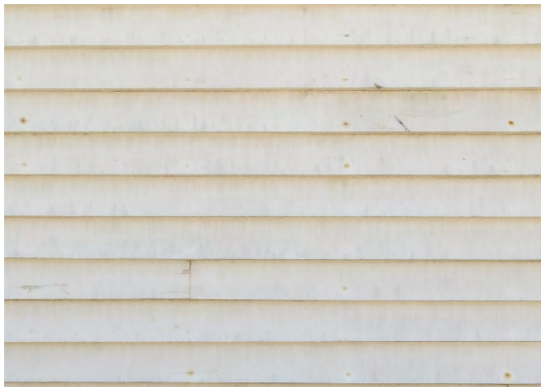
Figure 28. Oxidized non-galvanized nail heads are staining the siding. These areas should be filled and painted to prevent further corrosion and damage (photo: Garavaglia Architecture, Inc., April 2013).
