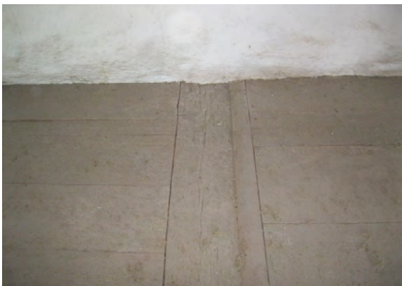
Figure A78. The large beams below correspond to perpendicular boards above. There appears to be ghosting from a former partition in this location.
