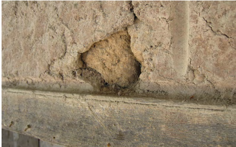
Figure 46. At an unknown time in the past, a decision was made to apply an adobe parge coat to the Servants' Quarters. This coat was then scored to resemble large adobe bricks. Now the layer is failing, sometimes spalling off in large sections to expose the original adobe beneath (photo: Garavaglia Architecture, Inc., April 2013).
