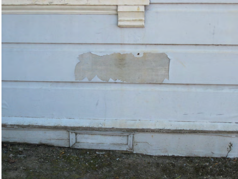
Figure 39. Paint finishes are failing on the Hotel Annex. An earlier, similar shade of blue is visible beneath the more recent latex paint (photo: Garavaglia Architecture, Inc., April 2013).
