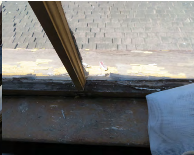
Figure 35. Paint is weathered and no longer protects the wood substrate. This image shows the interior and exterior surfaces of a windowsill on the second floor of the Kitchen Annex (photo: Garavaglia Architecture, Inc., April 2013).
