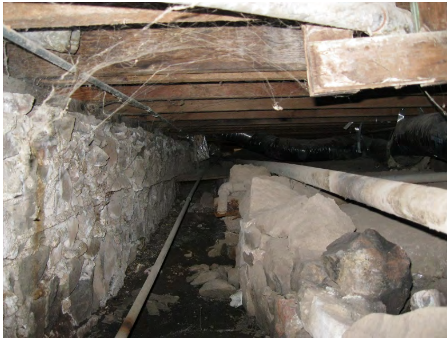
Figure 32. The Kitchen Annex has a large crawlspace and a rock foundation. A drainage pipe crosses under the building toward the street (photo: Garavaglia Architecture, Inc., April 2013).
