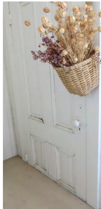
Figure 42. The east bathroom on the second floor of the Hotel Annex has been converted from part of a former bedroom. Here an original exterior door has been fixed shut and the floor raised to accommodate pipes to the fixtures.
