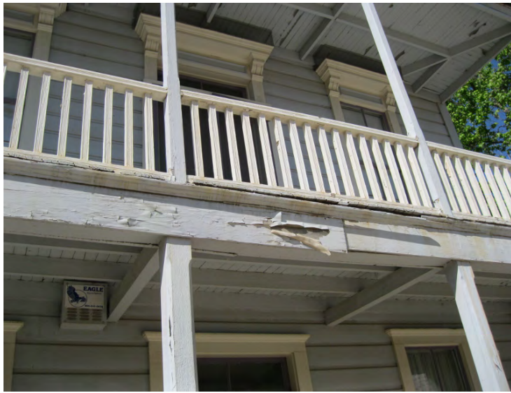
Figure 37. Failing finishes and material deterioration are more extreme on the second floor porch of the Hotel Annex than in other locations on the building. Here paint is failing, floorboards are warping, and the railing is loose and poorly attached (photo: Garavaglia Architecture, Inc., April 2013).
