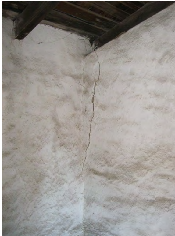
Figure 53. This is an example of the types of corner cracks found on the second floor of the Servants' Quarters.
