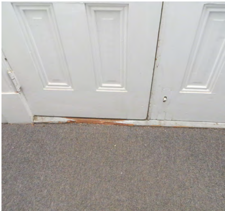
Figure 41. The front door of the Hotel Annex has a worn and damaged threshold. Otherwise, this assembly appears to be in good condition with several elements of original hardware still in place (both photos: Garavaglia Architecture, Inc., April 2013).
