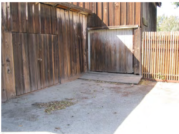
Figure A89. Detail the primary entrances to the two sections of the barn, looking northwest.
