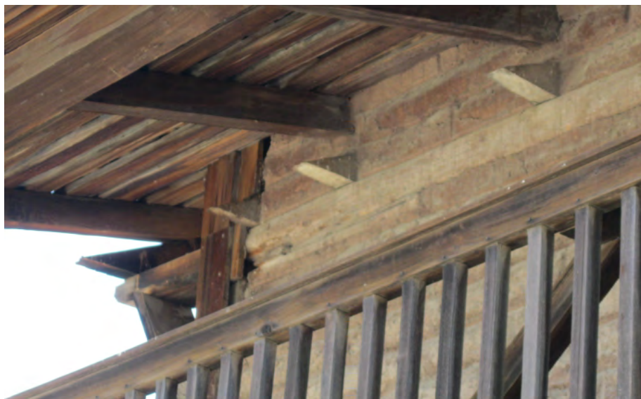
Figure 47. Birds are nesting in the south wall of the Servants' Quarters. Here a double layer of wood siding is filled with adobe and straw. The birds are getting into this interstitial space at the southwest corner (shown) (photo: Garavaglia Architecture, Inc., April 2013).
