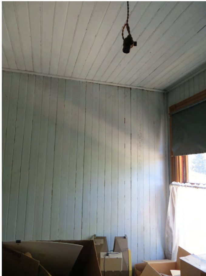
Figure 33. Leaks in the Kitchen Annex roof allow water to enter the finished rooms on the second floor. Here staining is visible where soiled water is washing down the face of the beadboard ceiling and walls (photo: Garavaglia Architecture, Inc., April 2013).
