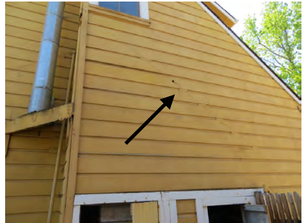
Figure A25. Detail of the stair enclosure on the north side. Note the ghosting of a shed roof that has been removed.
