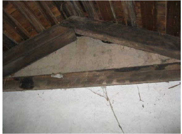
Figure A81. This cross wall has finished adobe bricks completely filling the void to the gable peak.
