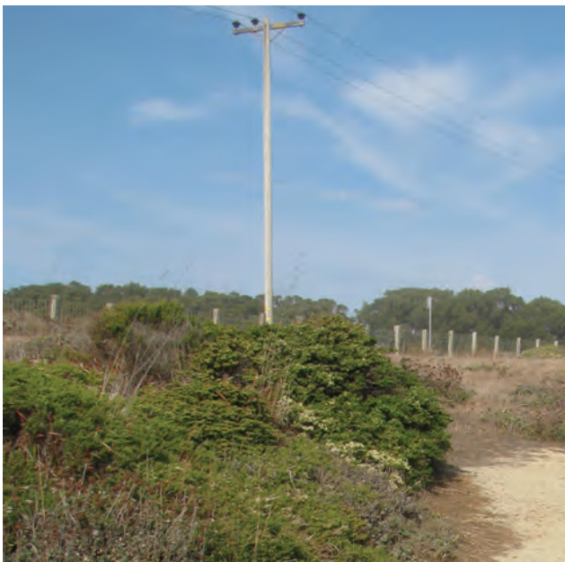
Utility Poles along Pigeon Point Road
