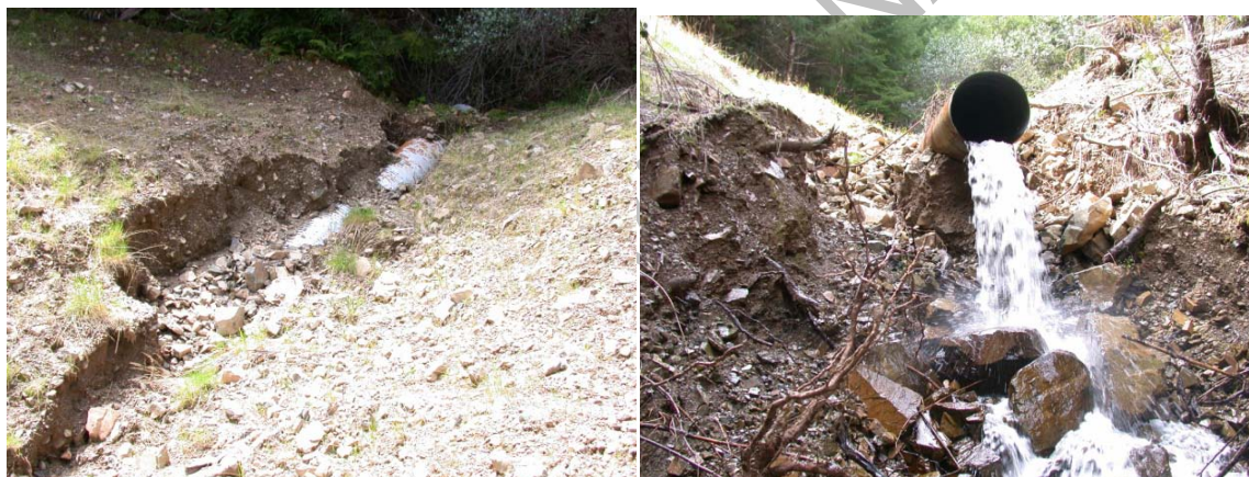
Figure 13. Chronic erosion of stream crossing fill on a partially removed (maintenance-free) crossing.
