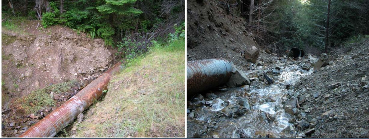
Figure 14. This partially removed stream crossing has subsequently failed and delivered sediment to the stream channel because of the ineffective method used to convert the crossing to maintenance-free status.
