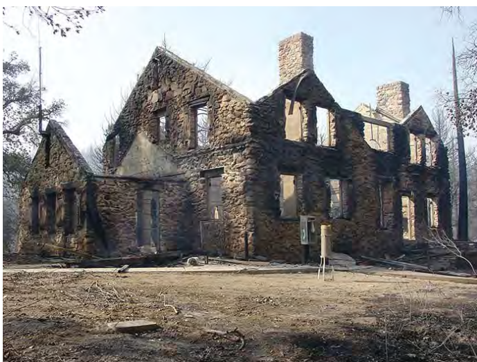
The Ralph M. Dyar House and former Park headquarters after the Cedar Fire
