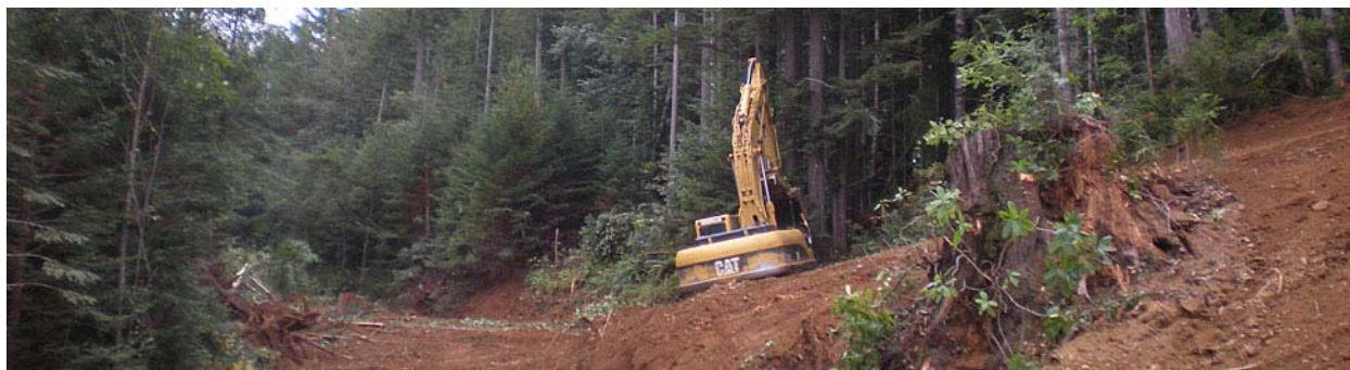
Road removal work at the Mill Creek Addition. Source: Photograph taken by AECOM in 2010.
