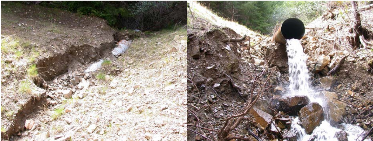
Figure 14. Chronic erosion of stream crossing fill on a partially removed (maintenance-free) crossing.
