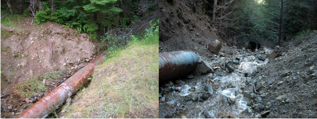
Figure 15. This partially removed stream crossing failed and delivered sediment to the stream channel because of the ineffective method used to convert the crossing to maintenance-free status.
