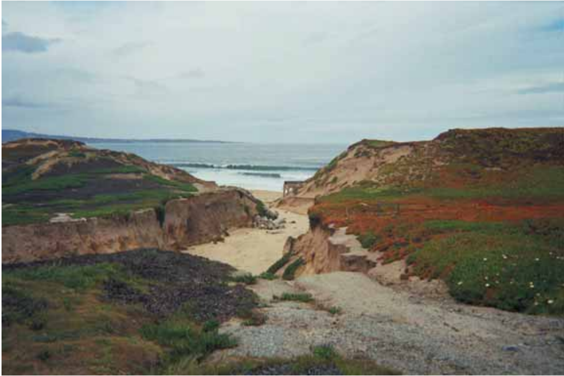
Erosion at Stormwater Outfall (with former outfall structure)
