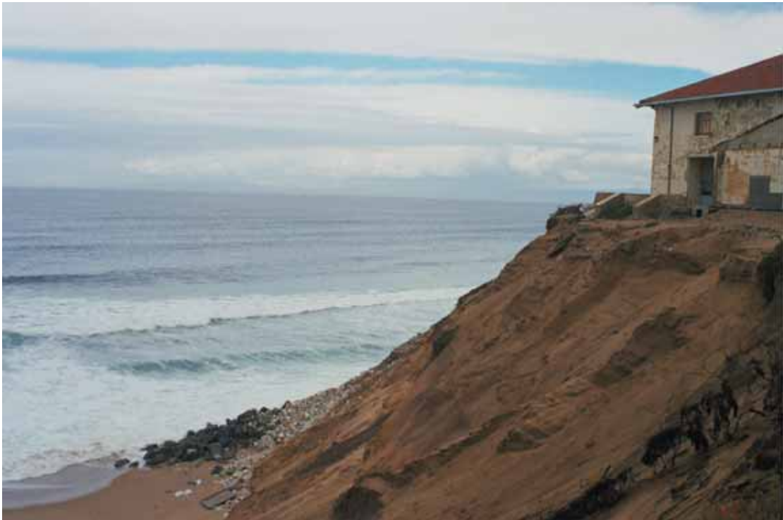
Coastal Erosion at former Stillwell Hall
