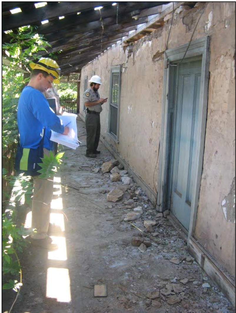
Image 15: State Park staff assesses earthquake damage at the Blue Wing Inn.
