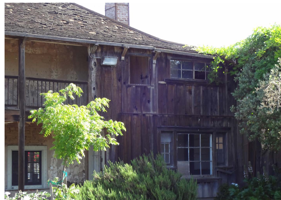
Photograph D: Blue Wing Inn, exterior at southeast corner. Area of proposed new egress stair & elevator. 2013.
