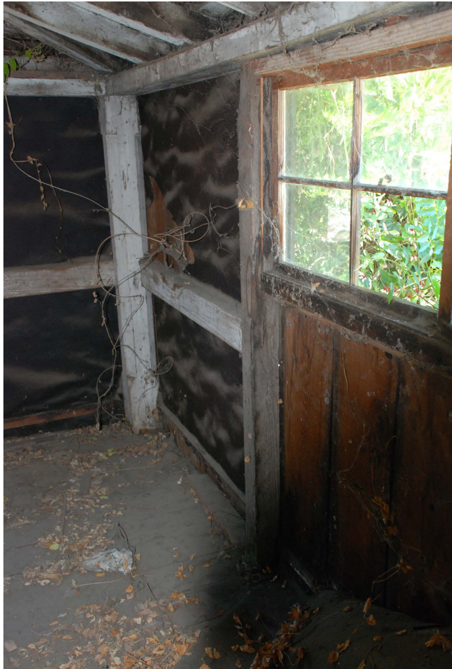
Photograph C: Blue Wing Inn, interior at second level porch at southwest corner. Area of proposed new egress stair & elevator. 2013.
