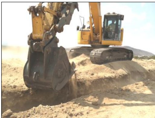
Adam Asche uses the excavator to gently shade the assembled pipeline to prevent any rocks that get pushed into the ditch during the backfilling process from breaking or cracking the pipeline.
