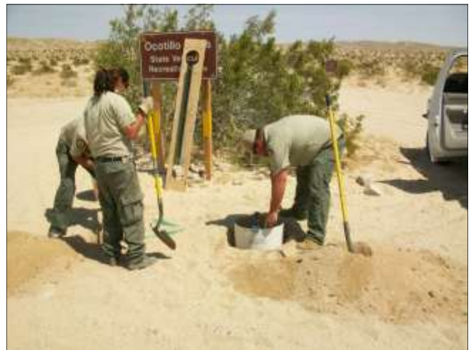
Ryan Walasek digs out the second post hole while Krystal Friel stands by as Josh McCue checks the concrete tube for level.
