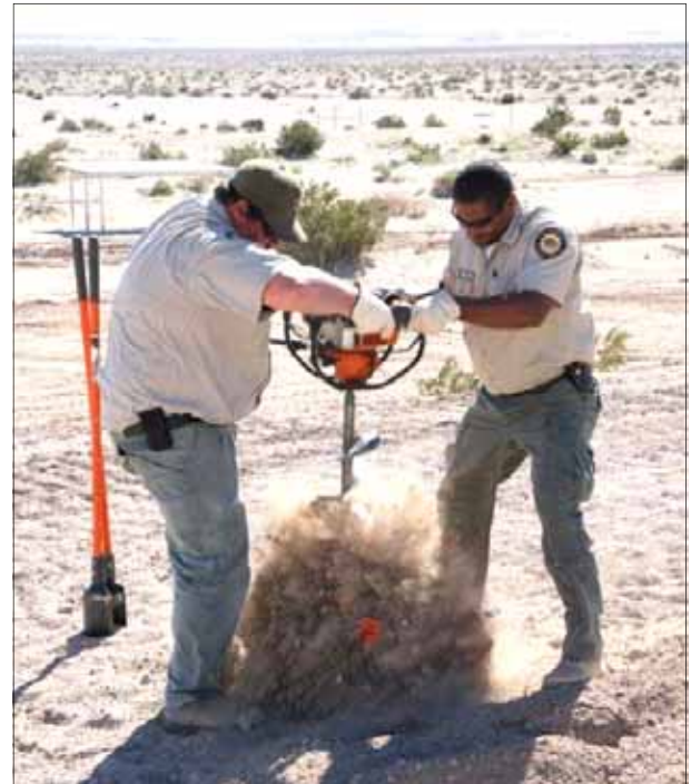
Dirt flies from the post hole as Joshua McCue and Anthony Beepath use a two-man auger to install a sign at the new Truckhaven 4x4 Obstacle Training Area.
