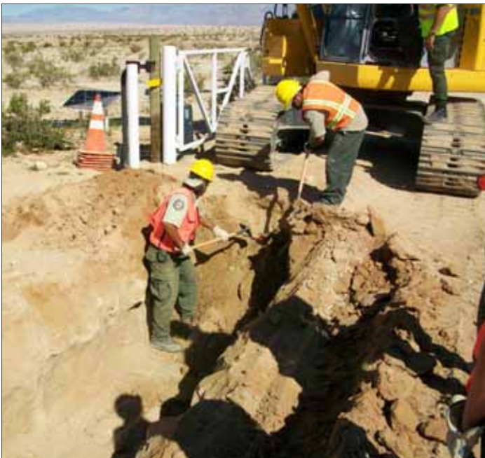
Martin Rubalcava and Cesar Casillas carefully hand dig around wires that crossed the new Toner phone line utility ditch.
