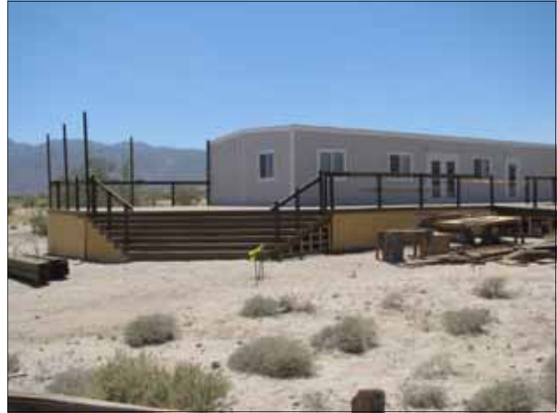
The Discovery Center gets a start on an ADA ramp. Skirting is also attached.
