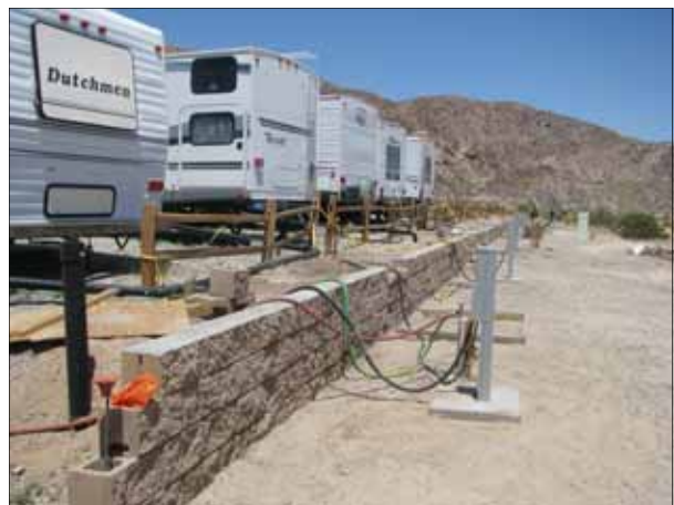
Block work continues on two retaining walls located at the rangers' parking area and the trailer resident area.
