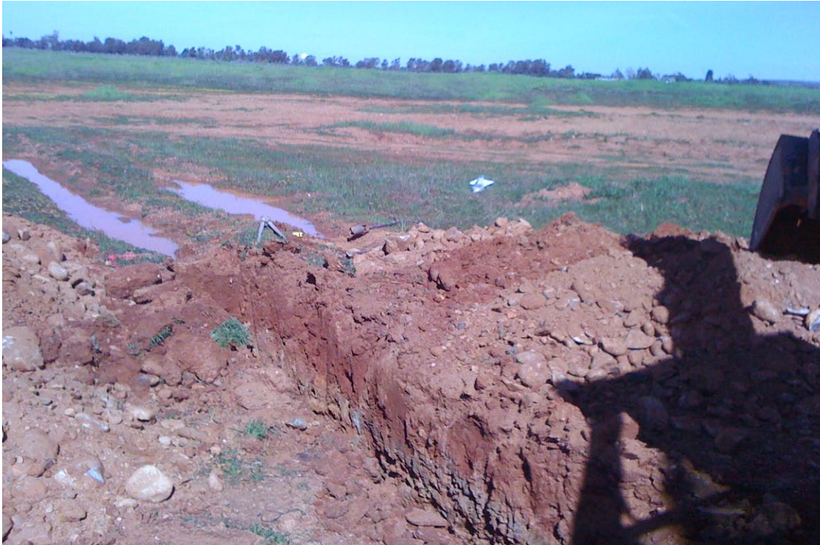
Photo No. 3 Standing Water from Recent Rain
