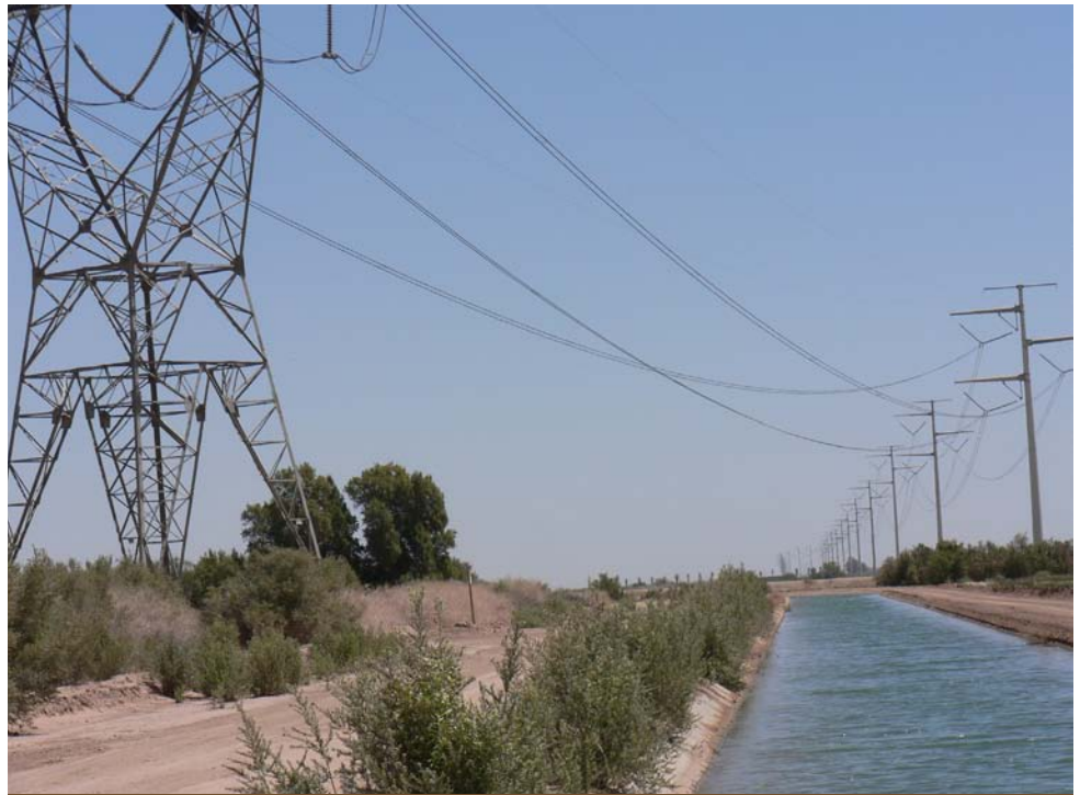
Transmission lines at the south end of the park.
