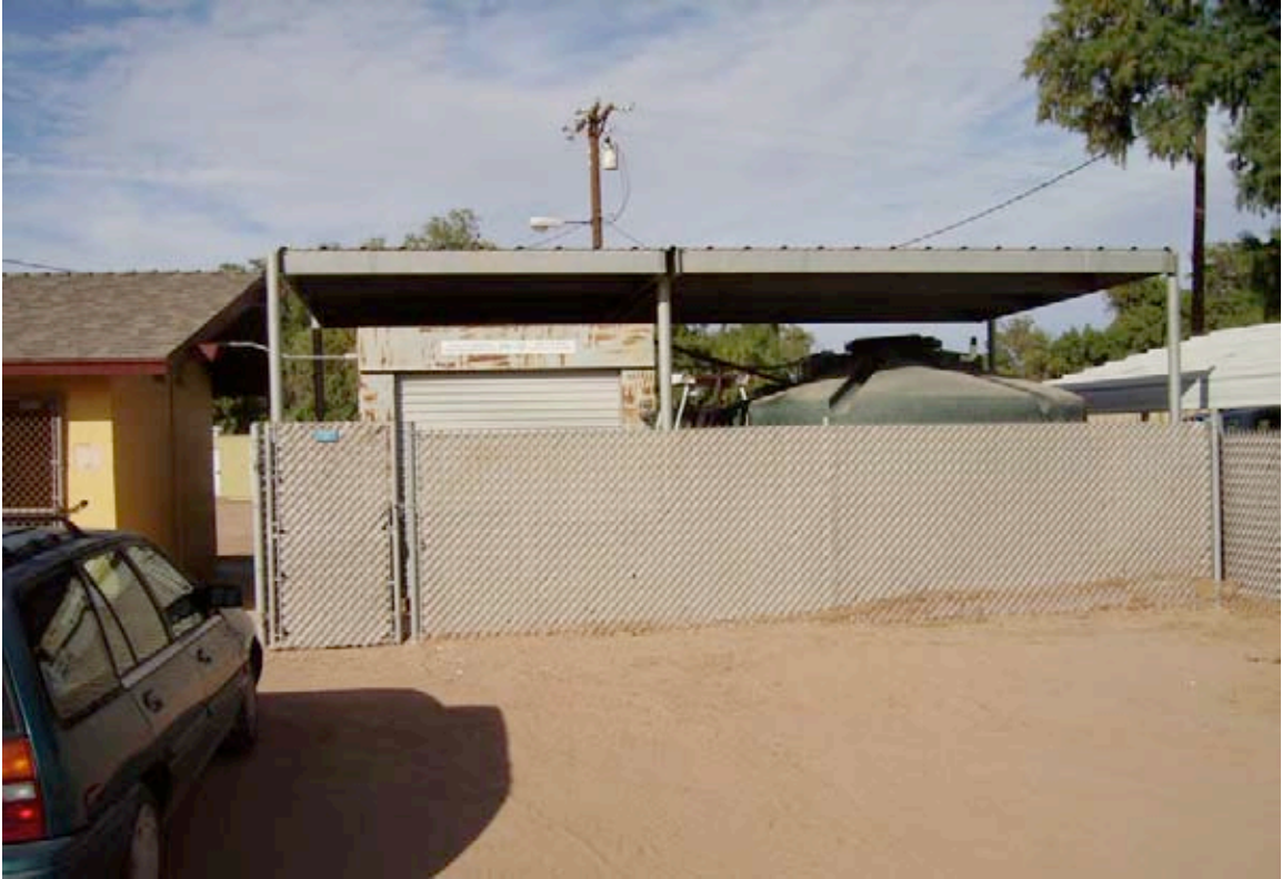
Photograph 7. View of water treatment unit, treats Colorado surface water from South Alamo Canal. Pole mounted transformer in distance near storage buildings.
