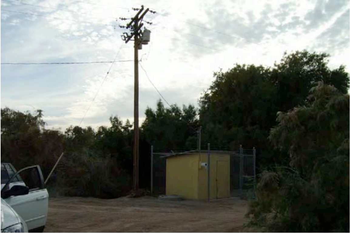
Photograph 15. View of electrical service with three pole-mounted transformers. Shed located for water intake to park.
