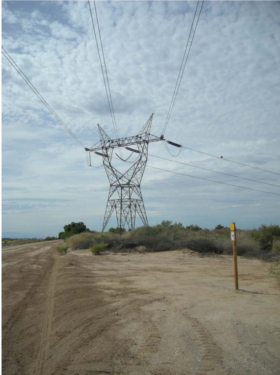
Photo 3.6-3. View of SDG&E electrical tower and overhead transmission lines
