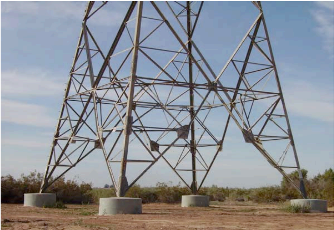
Photograph 12. View of power line support tower, note lack of climbing guards on legs.
