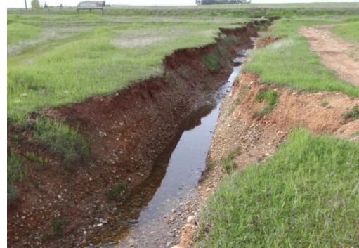
Drainage from southwest culvert under Larkin Rd.
