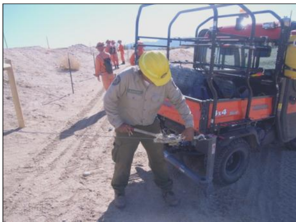
Left: Martin Rubalcava uses the come-a-long to keep tension on the fencing that the crew is installing to protect visitors from entering into a hazardous structure area.
