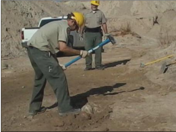
Left: While Pete Hernandez looks on, Ryan Walasek works on removing a rock protruding from the trail corridor.
