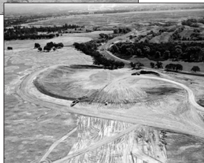
Overview of borrow area for Lake Oroville Dam; now Clay Pit SVRA
