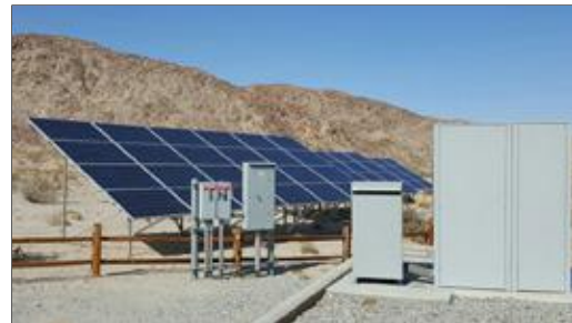
Solar panel system
