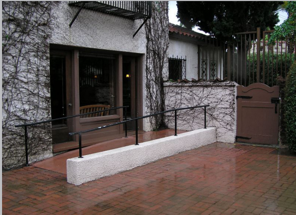
Wattles Mansion, Hollywood - Use of state grant funding for accessibility work, and building and garden restoration
