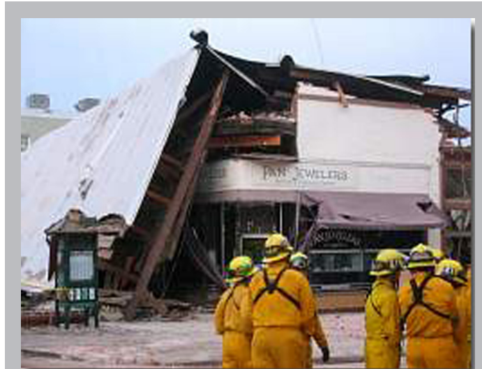
Acorn (Marrow) Building, Paso Robles - Built in 1892, this historic unreinforced masonry building collapsed December 22, 2003 during a 6.5 magnitude earthquake. 82 downtown buildings, some of them historic but not listed, were also damaged by the quake.
