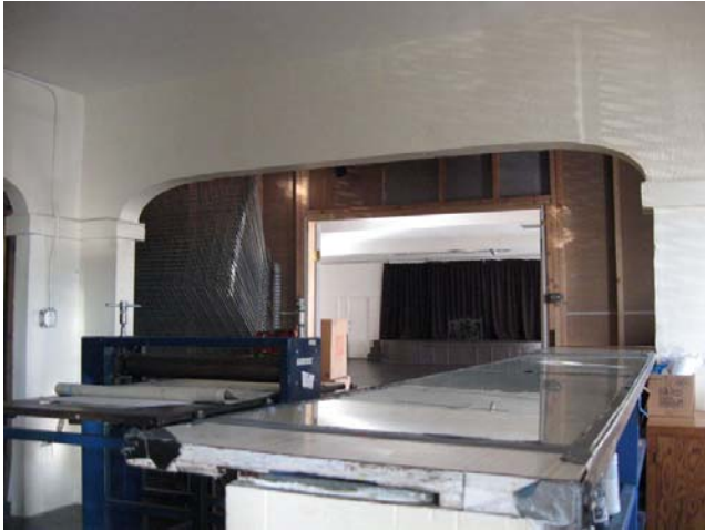
Arched openings and counter looking toward multi-purpose room. (Edgar Garcia) Arched openings and counter at rear of multi-purpose room
