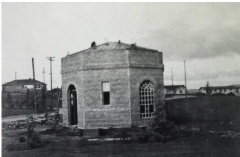
Figure 4: Memorial Hall under construction, looking north, circa 1924. Photo from the collection of the Crockett Museum and Historical Society.
