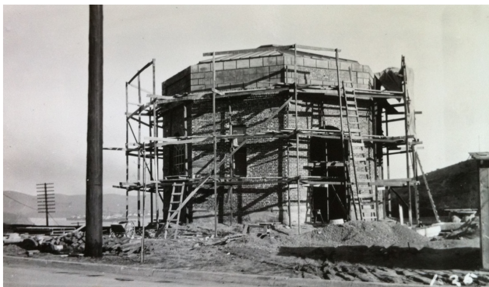
Figure 6: Memorial Hall under construction circa 1924. Note the scored plaster is being applied. Photo from the collection of the Crockett Museum and Historical Society.
