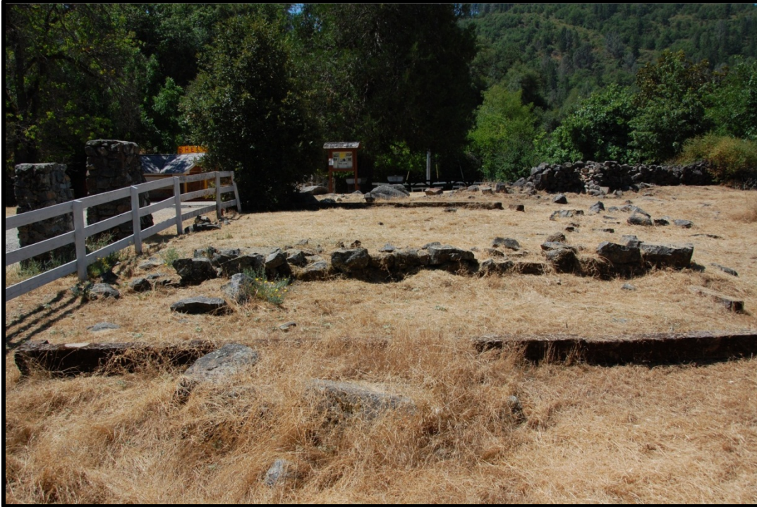
Photo 12. Dairy barn and tack shed foundations from the north. Photographed by David Anderson, June 2012.
