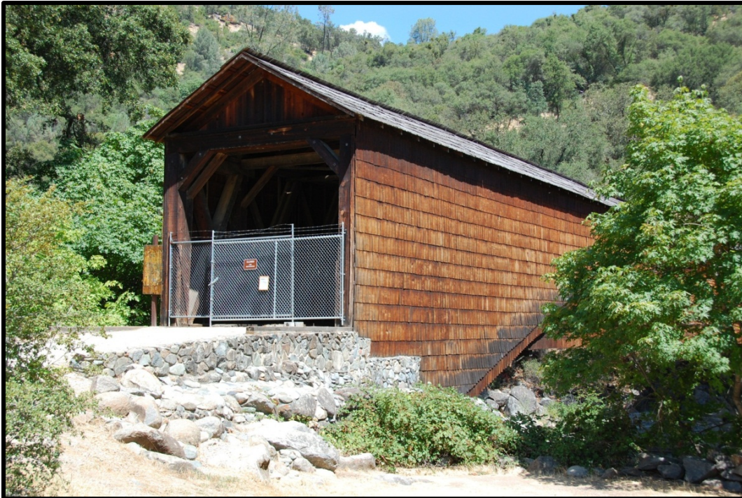
Photo 2. Oblique view of south entrance, also showing east side of bridge. Photographed by David Anderson, June 2012.
