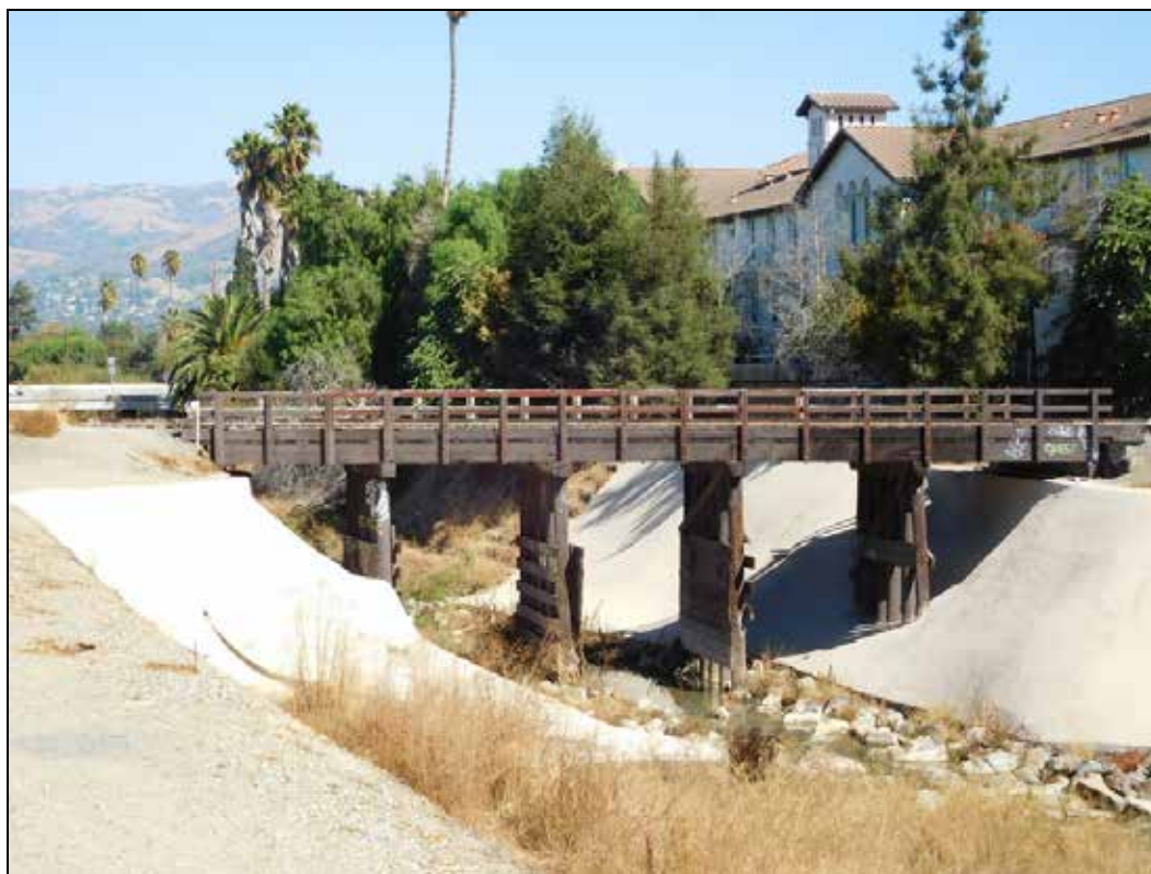
Figure 14. Western Pacific West San Jose Spur pile-bent trestle over Silver Creek, San Jose, California. Note the replaced abutments and concrete installed on embankments, both of which impact the integrity of this example.
