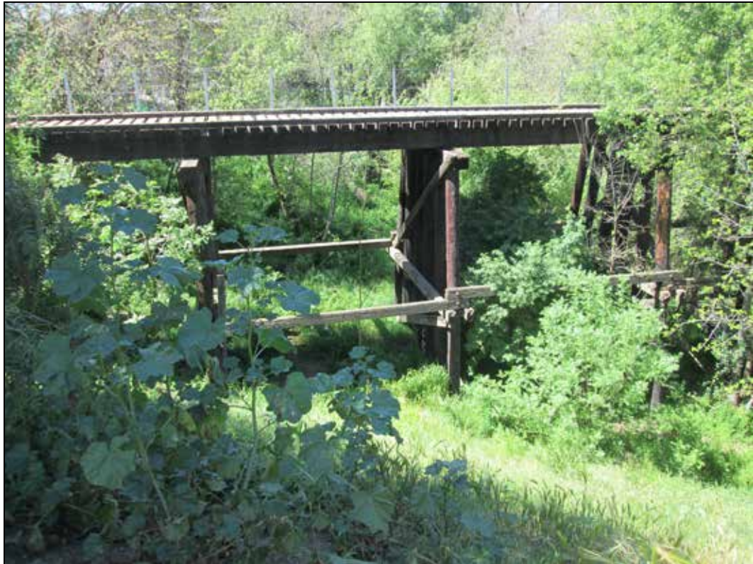
Figure 12. Western Pacific Railroad pile-bent trestle bridge over Coyote Creek, near Story Road, San Jose, one of four (including the Willow Glen Trestle) extant pile-bent trestle bridges in Santa Clara County.
