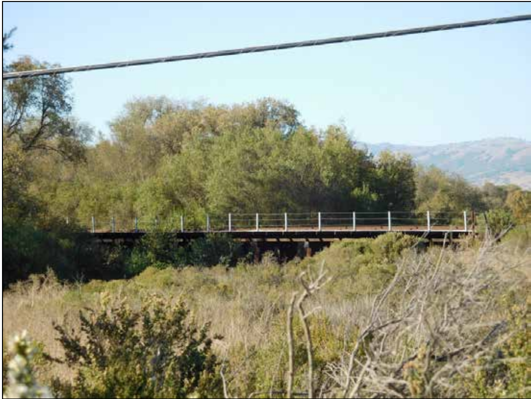
Figure 13. Southern Pacific pile-bent trestle over Pajaro River, near San Benito County line, on active railroad line and inaccessible to the public.
