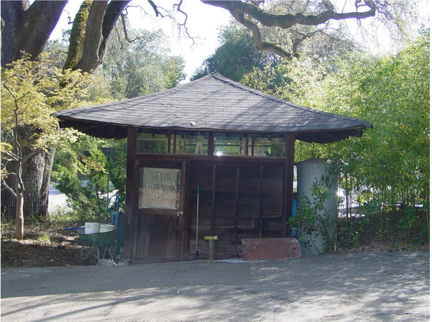
View east at Well/Pump House located in service area west of parking lot.
