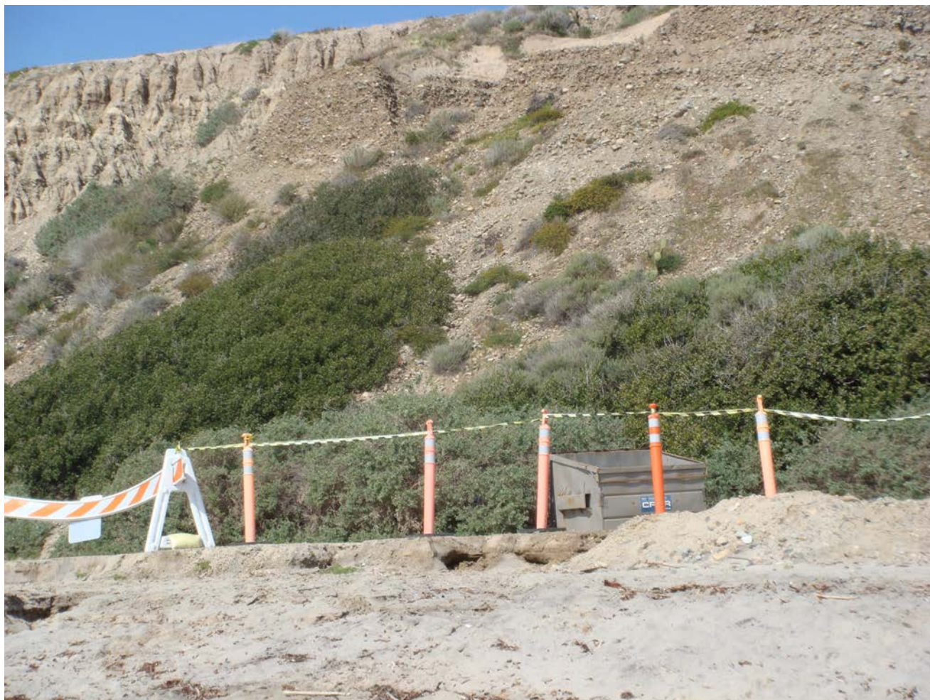
CA_San Diego County_Trestles Historic District_0030 Dog Patch, bluff, natural drainage, wash out at south end of parking area, looking northeast
