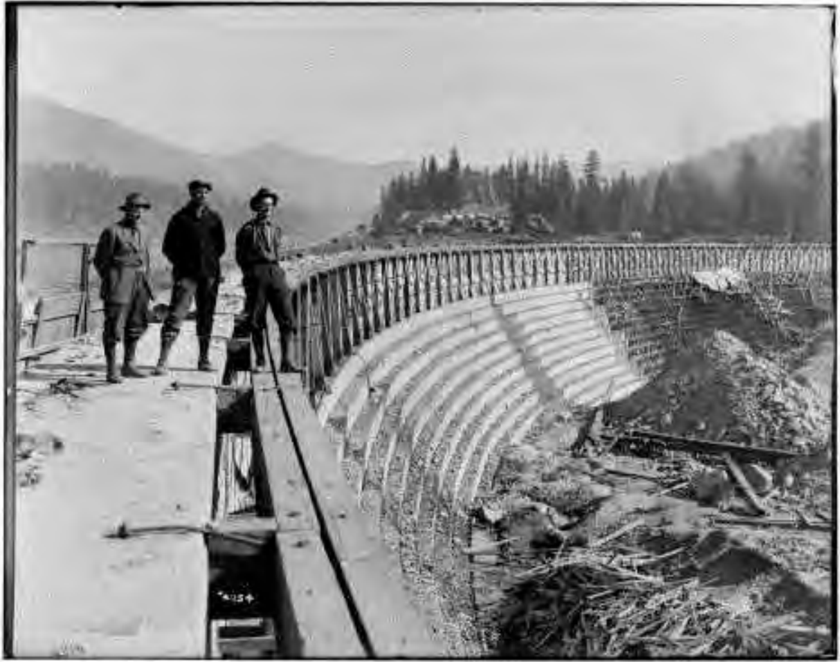
Figure 4: Huntington Lake Dam No. 2 showing engineers on top of dam during construction for the raising of the dam in 1917, man on right appears to be David Redinger. Image No. SCE-02-04754, Huntington Digital Library.
