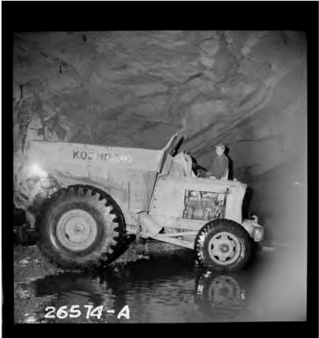
Figure 60: Repairs to Ward Tunnel, GM Dumpster Truck 1945. Image No. SCE-02-26574A, Huntington Digital Library.
