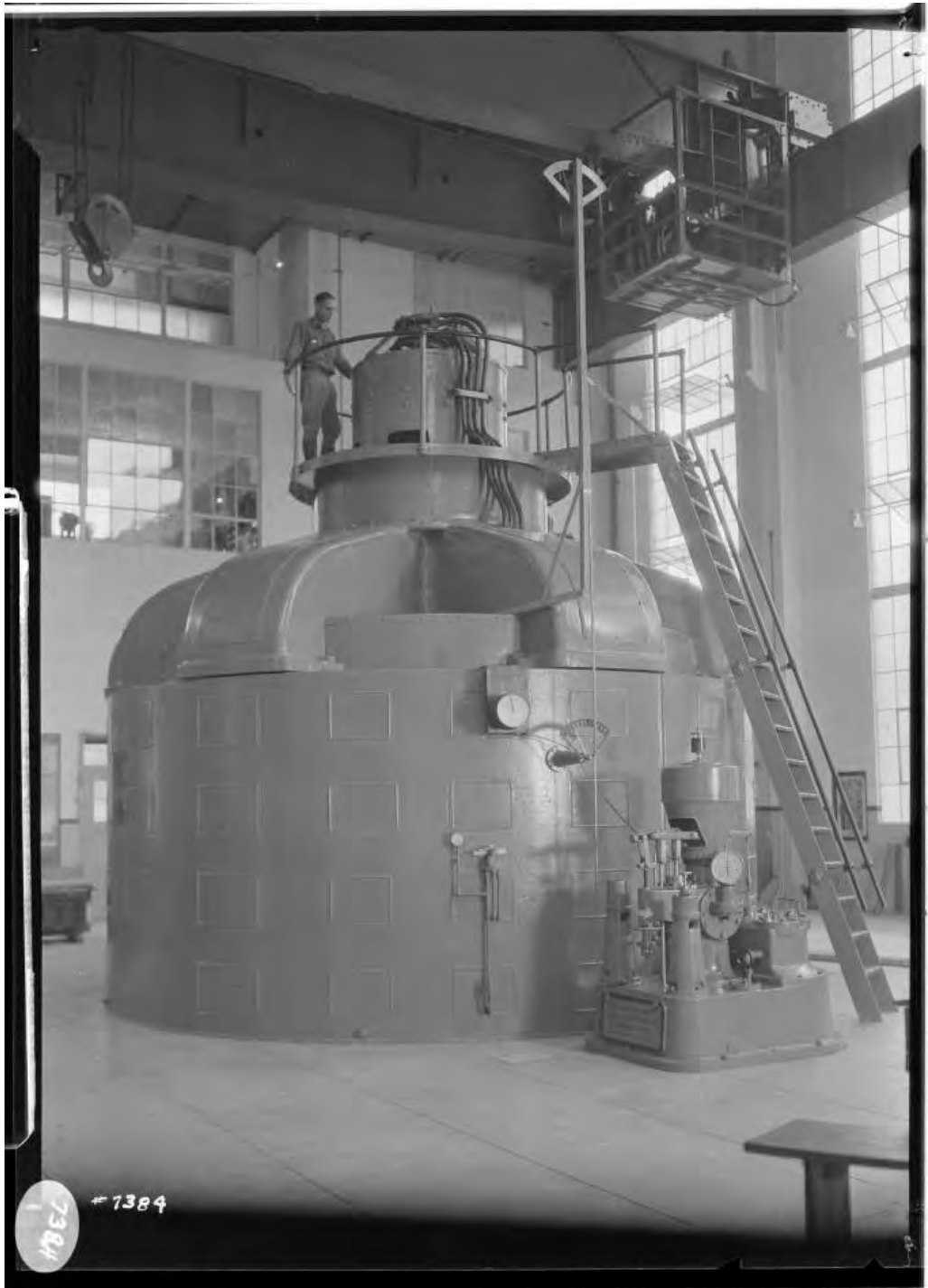
Figure 40: Powerhouse No. 8 Francis Type Turbine and Generator, 1921. Image No. SCE-02-07384, Huntington Digital Library.
