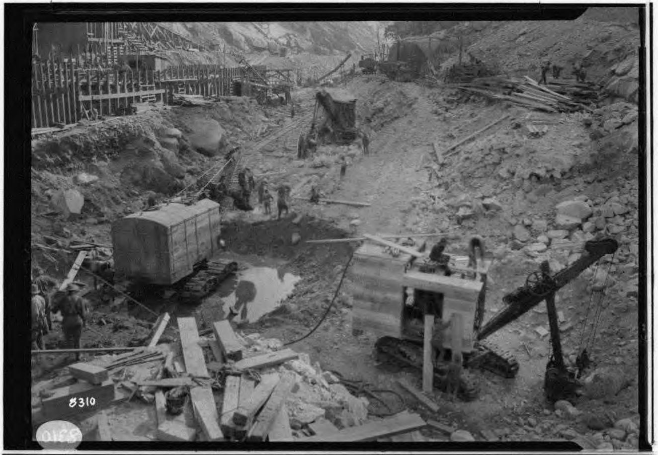
Figure 46: Excavation for Dam No. 6 in the San Joaquin River, 1922. Image No. SCE-02-08310, Huntington Digital Library.
