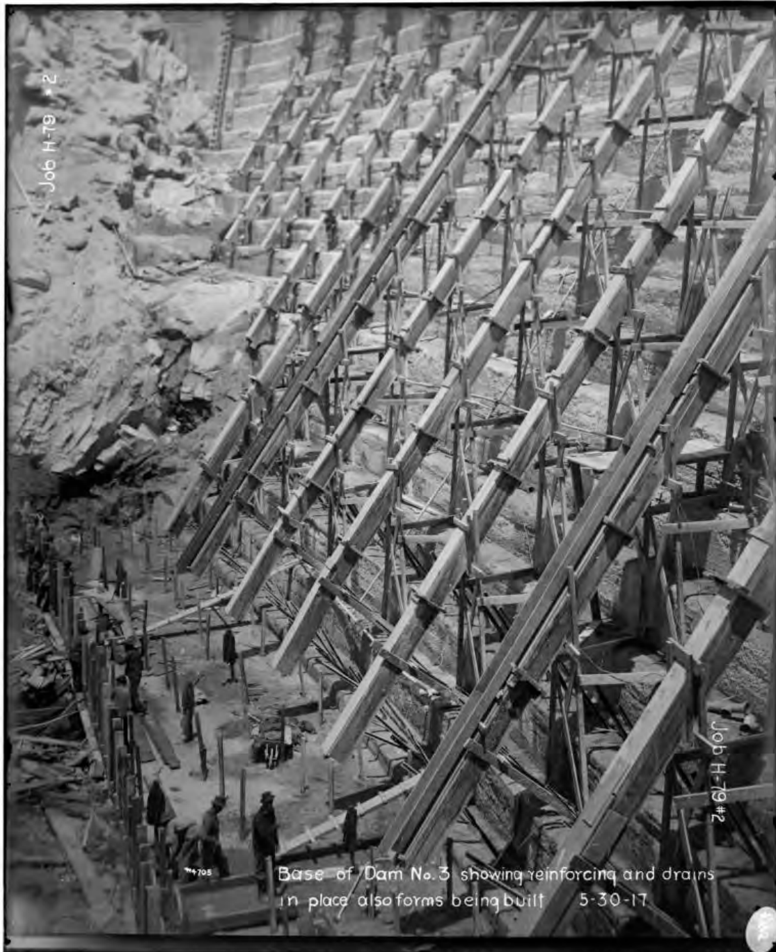
Figure 6: Huntington Lake Dam No. 3, 1917. Image depicts forms, reinforcing, and drains for raising of dam. Image No. SCE-02-04705, Huntington Digital Library.
