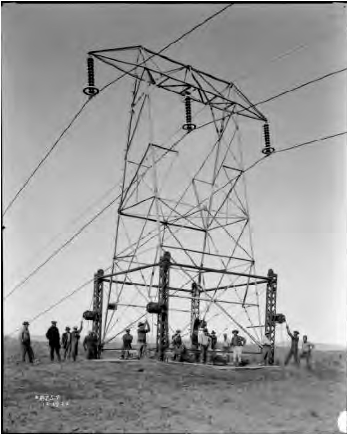
Figure 91: Raising Big Creek East and West Transmission Lines for 220 kV, 1922. Image No. SCE-02-08257, Huntington Digital Library.
