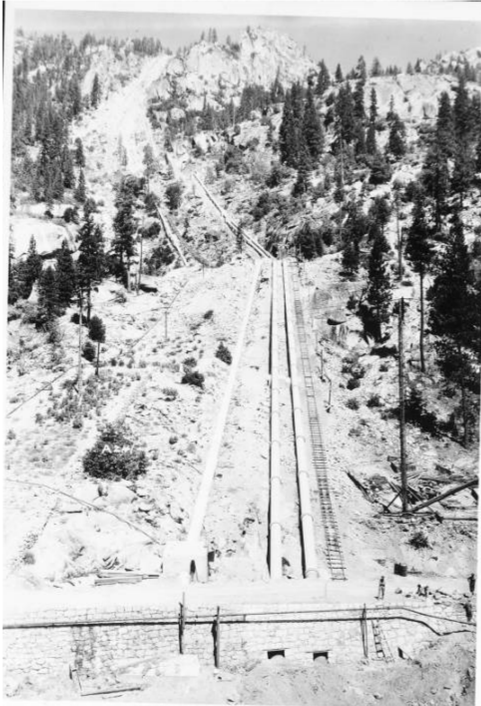
Figure 120: Incline No. 1 from Powerhouse No. 1 roof, 1913. Call No. Stone & Webster, 13-Vol. 028, PO35, Huntington Digital Library.
