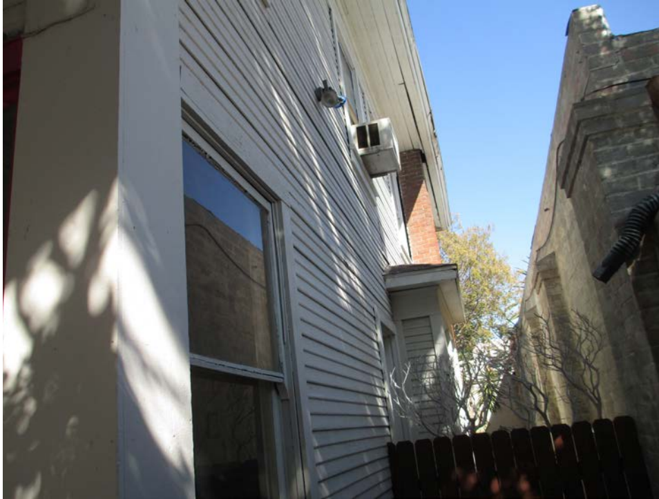
17 of 30. Exterior: Partial view of south façade, Hollywood School for Girls abutting Woman's Club of Hollywood building, view east
