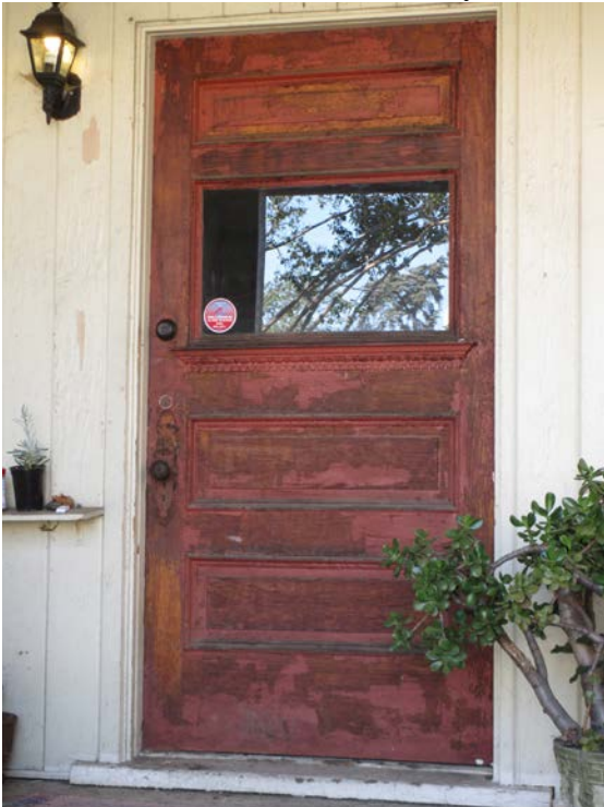
16 of 30. Exterior: Detail of Hollywood School for Girls headmistress' quarters, view west
