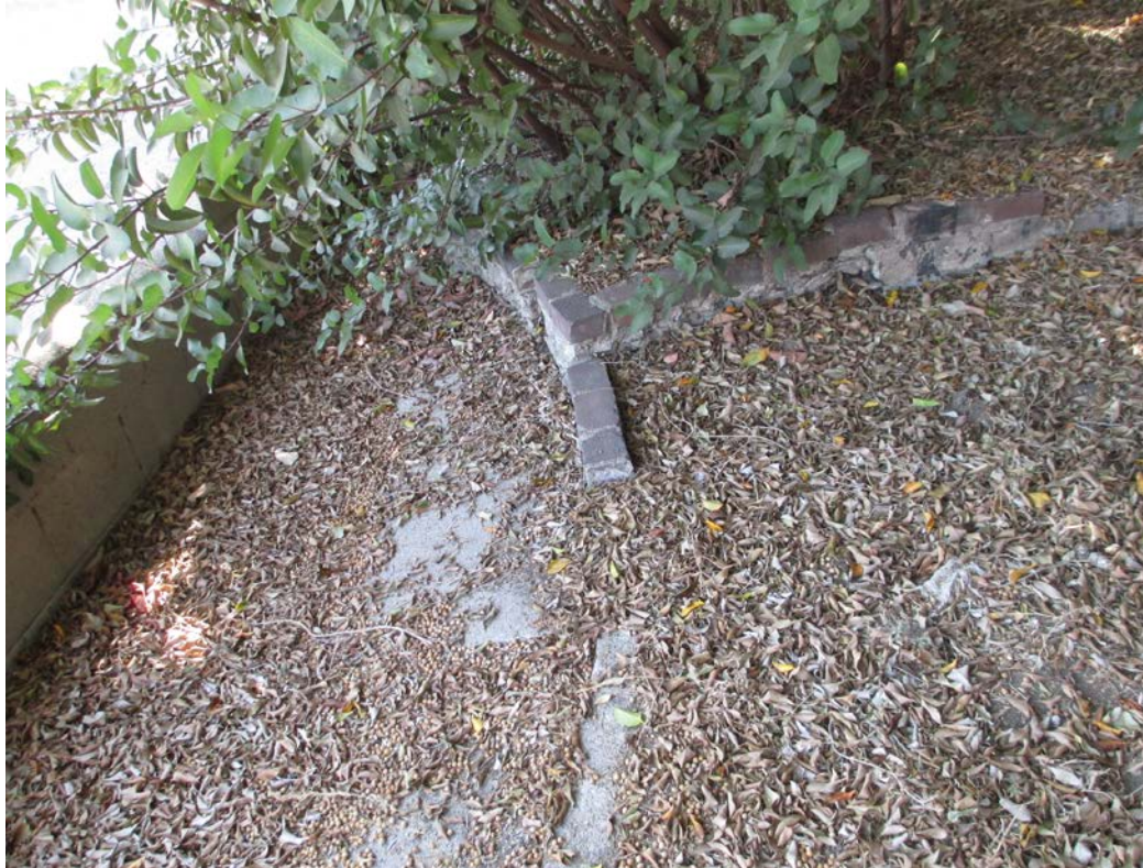
29 of 30. Exterior: Footing of one of original Hollywood School for Girls cottages
