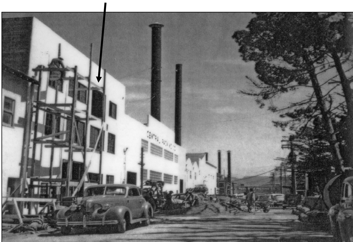
Figure 4. 1945 view of west façade of Aeneas Cannery building under construction. Note that the warehouse building and crossover have not been constructed yet. The large opening shown with an arrow is where the crossover will link to the cannery building. (Courtesy of the Pat Hathaway Collection of Historical Views)
