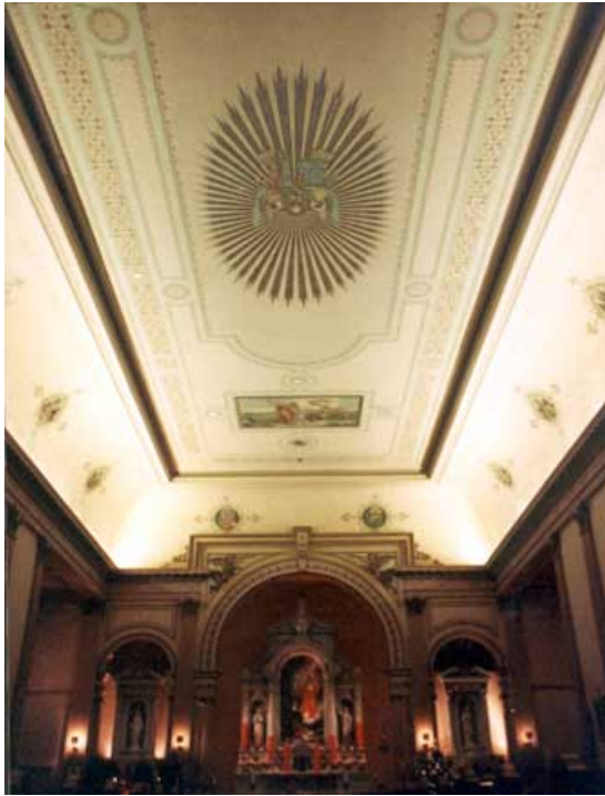
FIGURE 26. NAVE CEILING BEFORE HANGING OF SAFETY NETTING IN 1989 (PHOTO 2005, COURTESY KATHERINE PETRIN).
