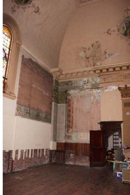
FIGURE 20: CHURCH: CHOIR LOFT, NORTHWEST CORNER AND DOOR TO STAIRS, SHOWING FINISH MATERIALS AND DECORATIVE TREATMENTS, 2016.
